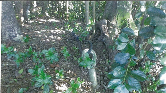
Slope Stabilization Anchor and cables on north side of property along Kūhiō Highway
