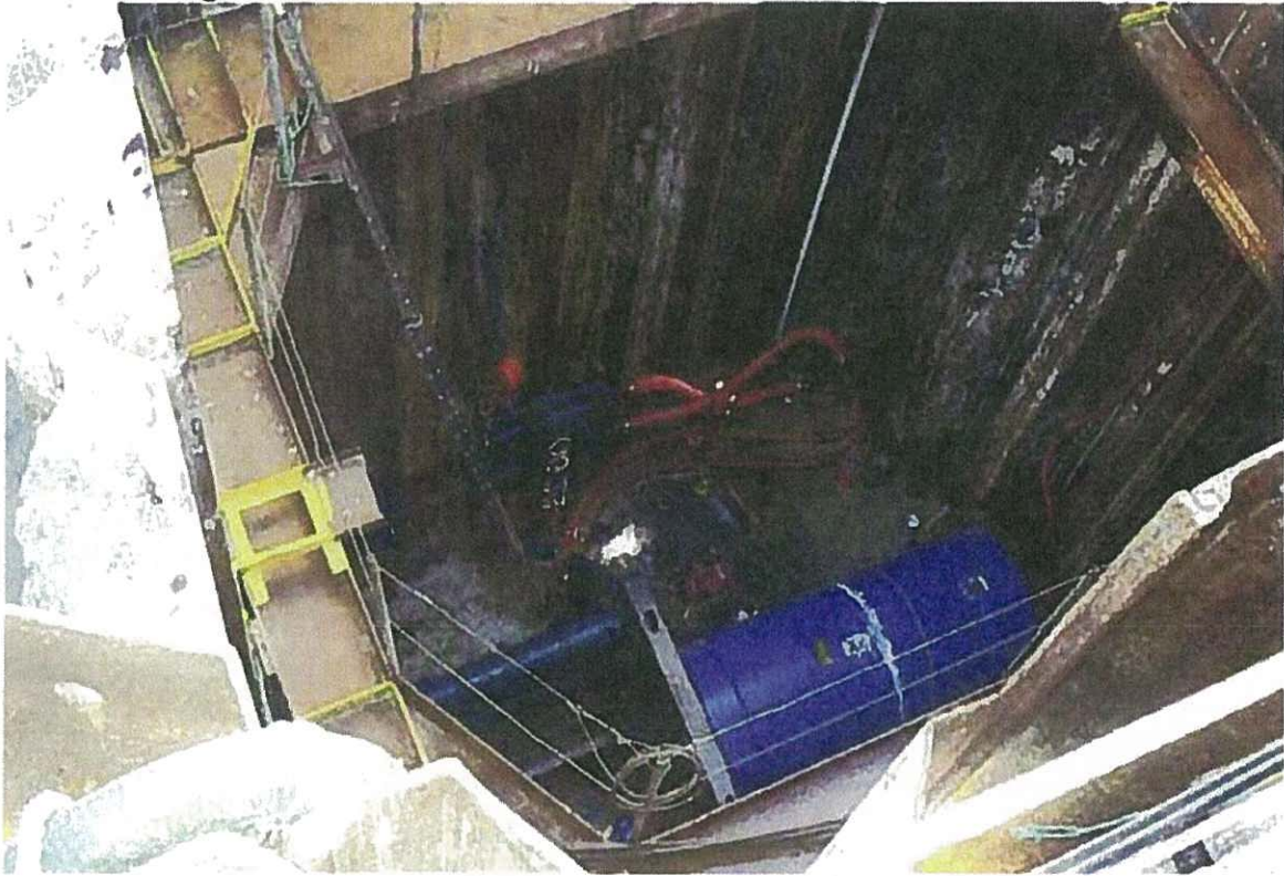
Sample of Micro-tunnel Shaft
