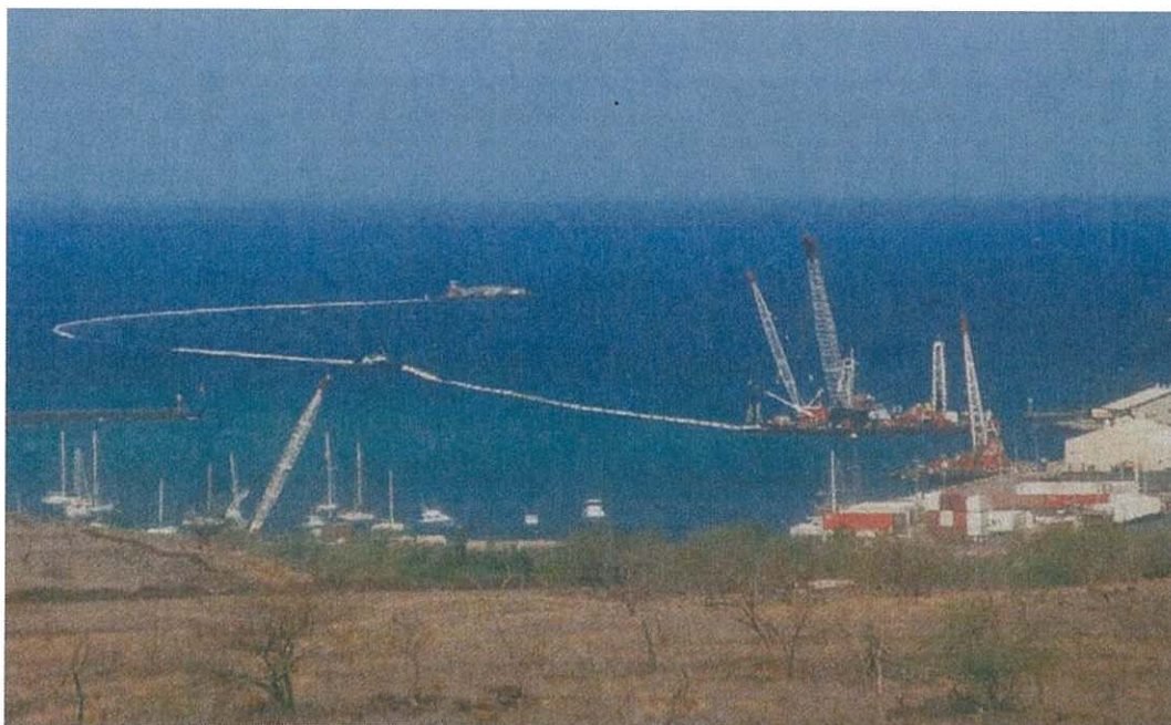
Photo 6. Example of fully assembled NELHA 55-inch Pipe Being Towed From Kawaihae Harbor Source: Makai Ocean Engineering, Inc. ( https://www.makai.com/ )
