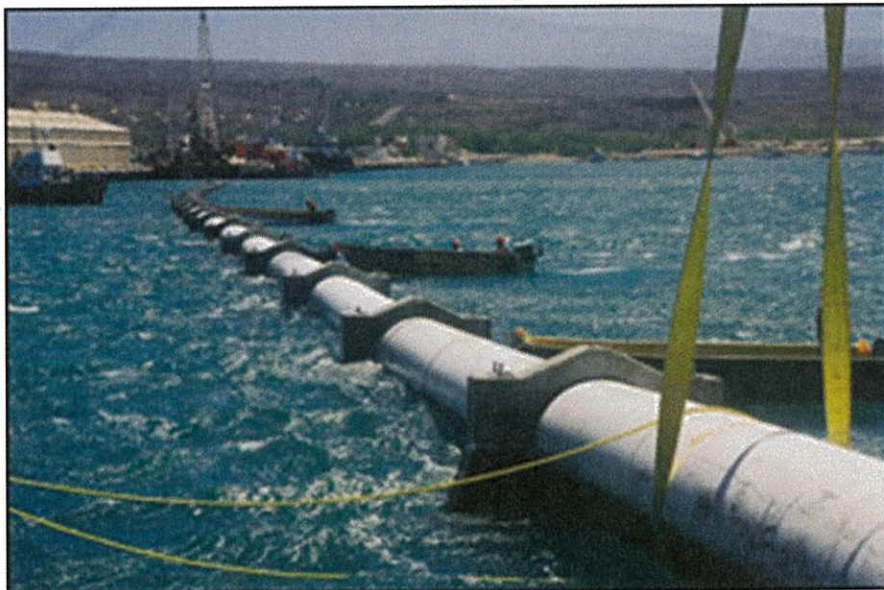
Photo 4. Example of a single 1.4 m (55") diameter NELHA deep-water intake pipeline during assembly. Source: Makai Ocean Engineering, Inc. ( https://www.makai.com/ )
