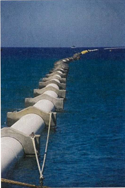
Photo 3. Example of single 1.4 m (55") diameter NELHA deep-water intake pipeline during assembly. Source: Makai Ocean Engineering, Inc. ( https://www.makai.com/ )
