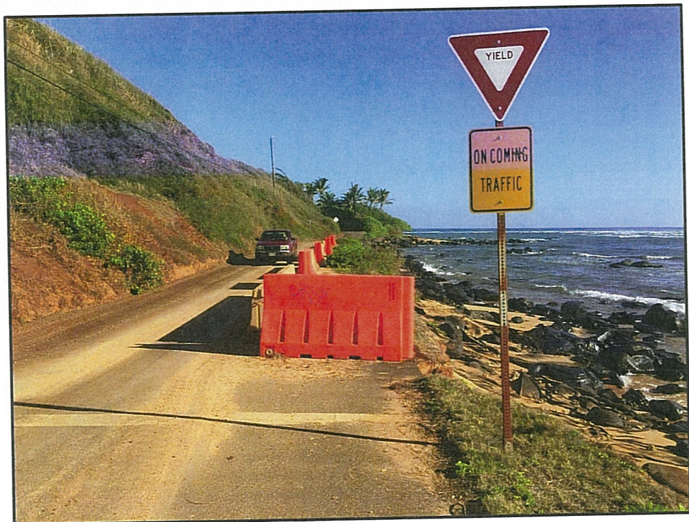
Figure 4. Photograph looking north along the damaged road.
