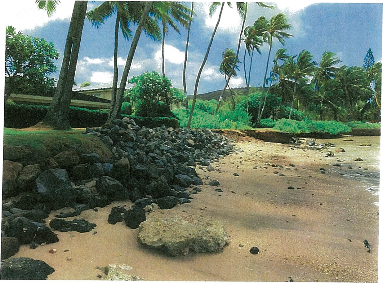
Figure 5 - Completed Revetment Placed Along Scarp Seaward of Residential Parcel and Located on and Seaward of Subject Beach Reserve Parcel, Facing Southeast
