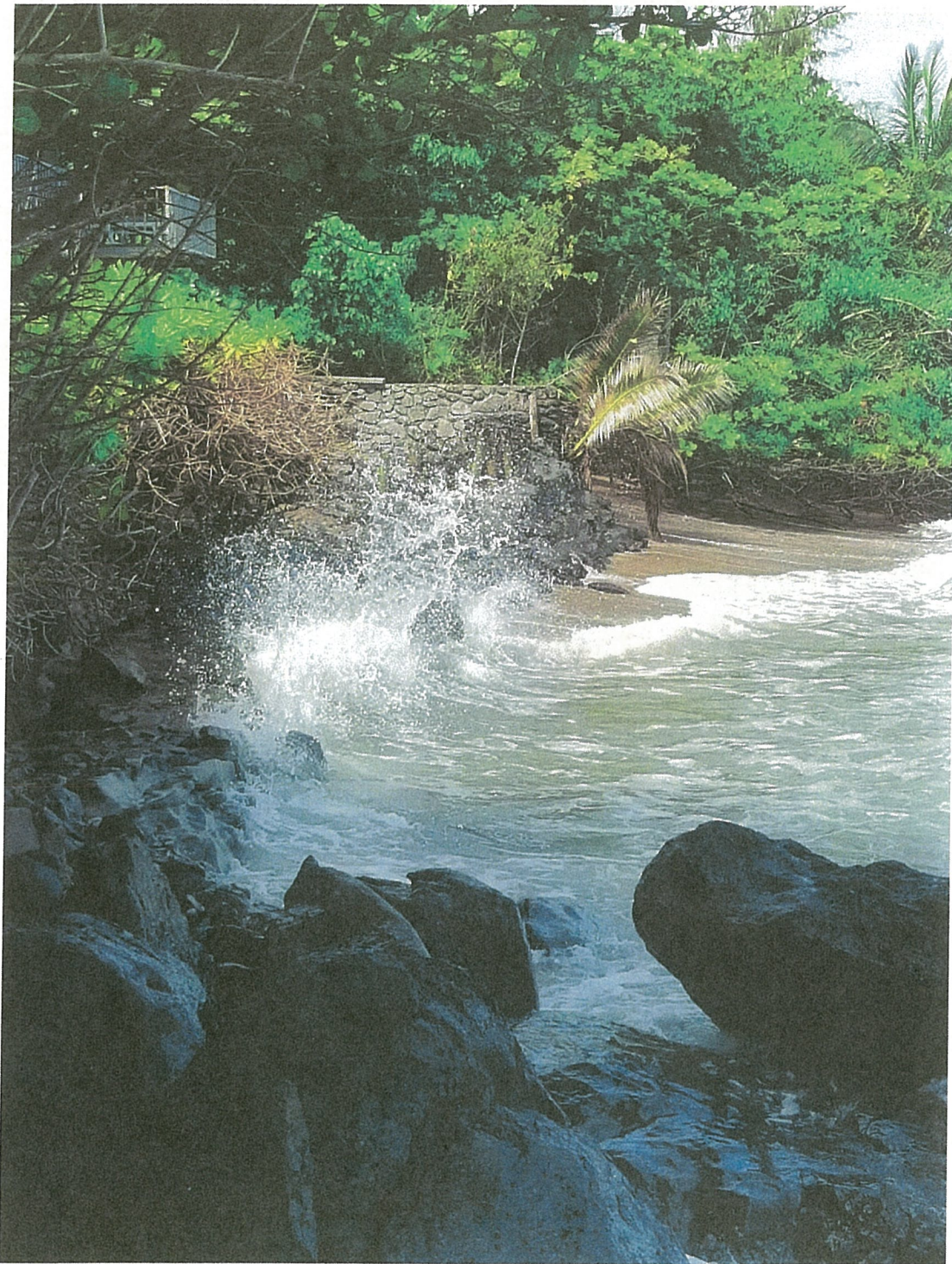
Figure 3 – Waves Washing Over Lower Section of Seawall
