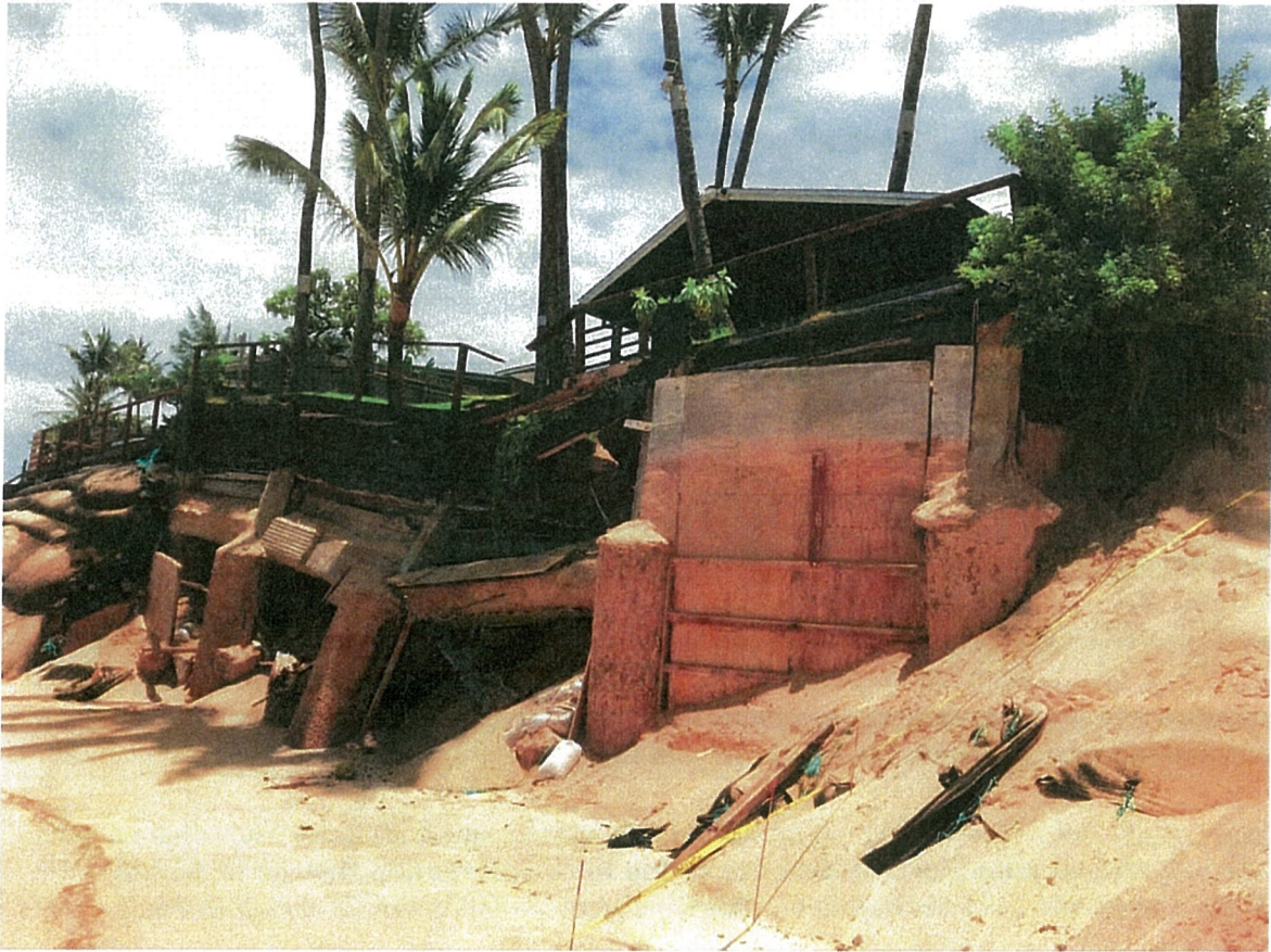
Figure 12 – July 28, 2020 Photo Showing Damaged Seawall
