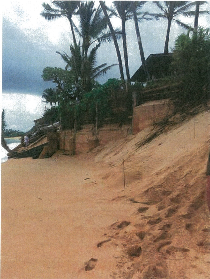
Figure 11 – September 17, 2018 Photo Showing Existing Condition Following an Erosion Event
