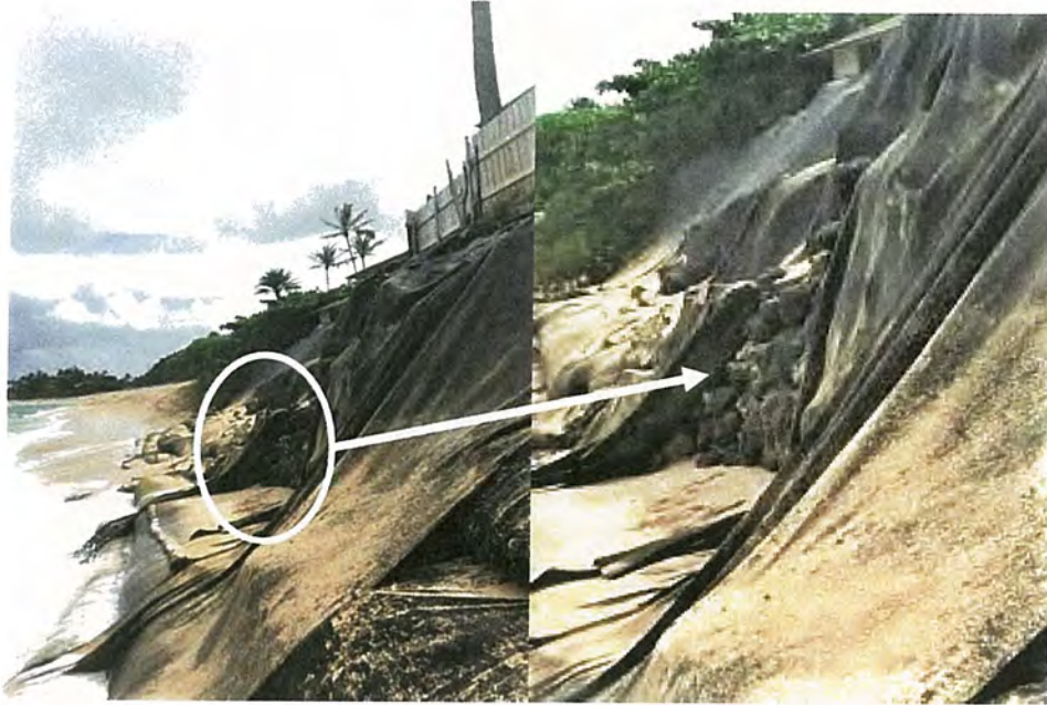
Figure 9: September 17, 2018 Photo Showing Damaged Temporary Erosion Control Structure with Rocks & Mortar Underneath Erosion Fabric
