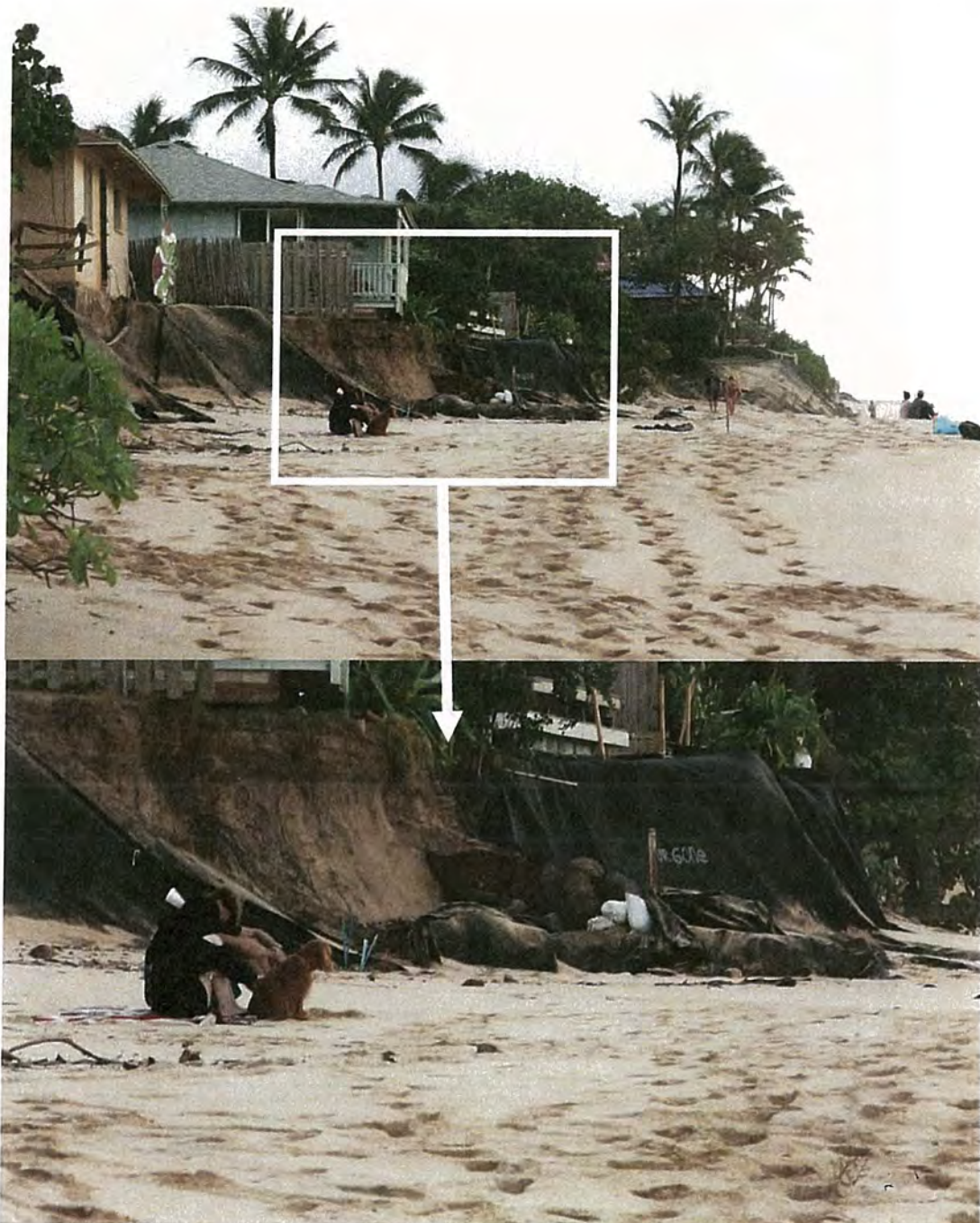
Figure 16: December 7, 2020 Photo Showing Dynamic Beach and Partially Covered Unauthorized Rock Revetment and Erosion Control Materials
