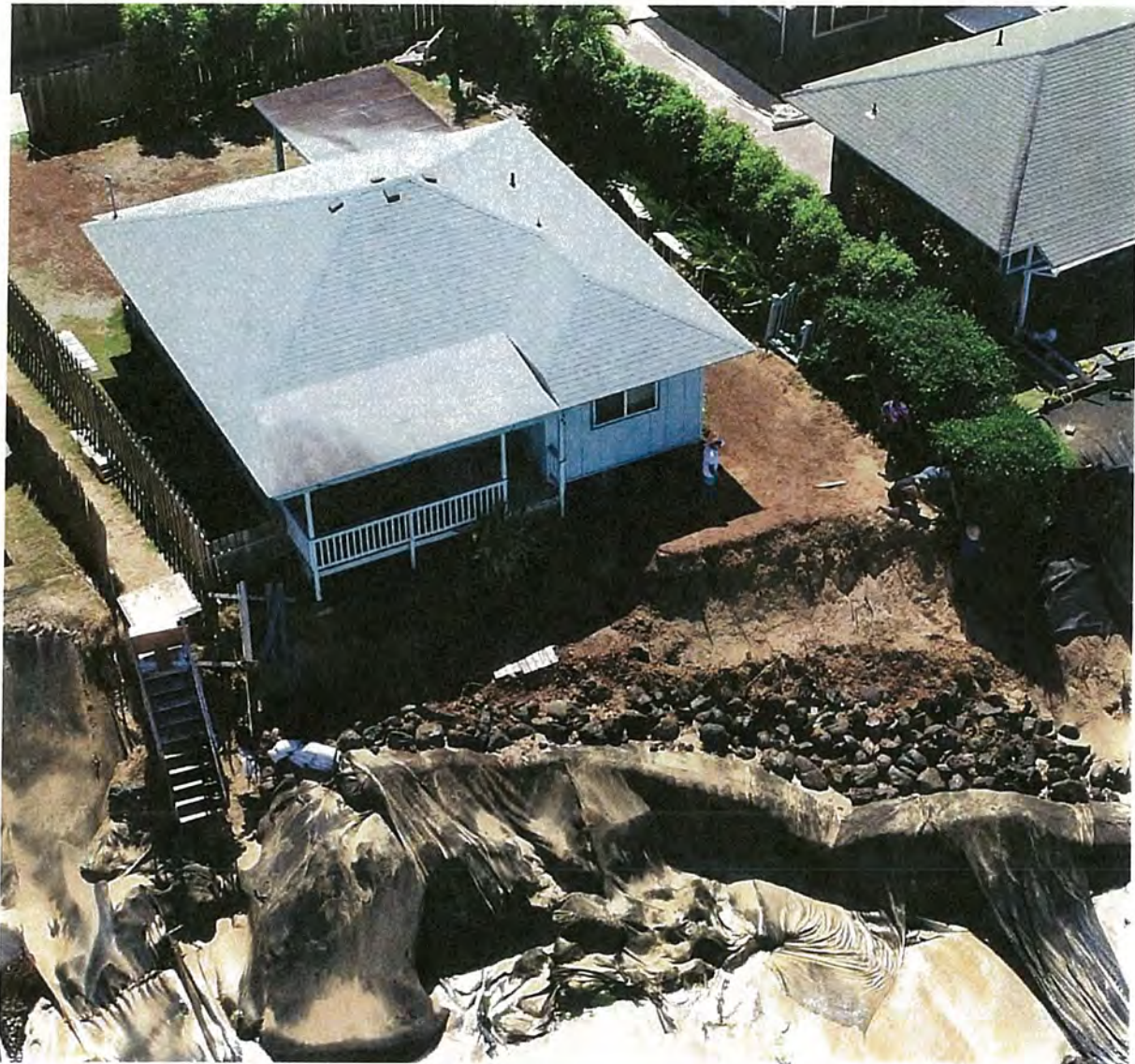
Figure 14: September 30, 2020 OCCL Site Visit Photo Showing Unauthorized Work & Makeshift Rock Revetment
