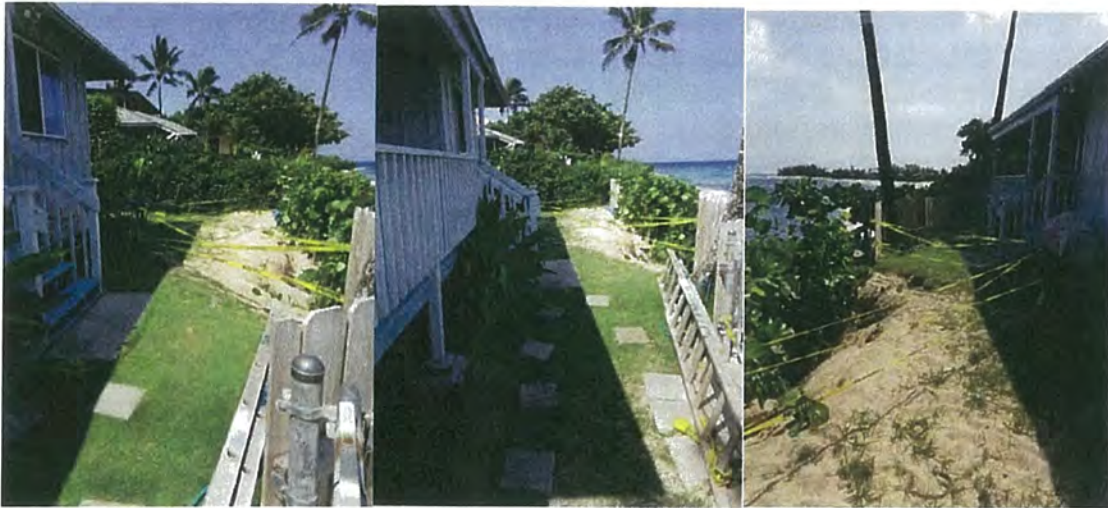
Figure 7: July 2018 Photo Showing Shoreline Area & Emergency Situation
