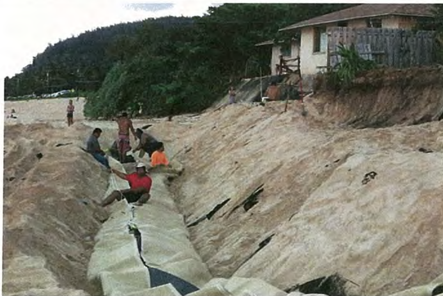
Figure 20: December 10, 2020 Photo Showing Unauthorized Work and Installation of Large Sand-Filled Burrito
