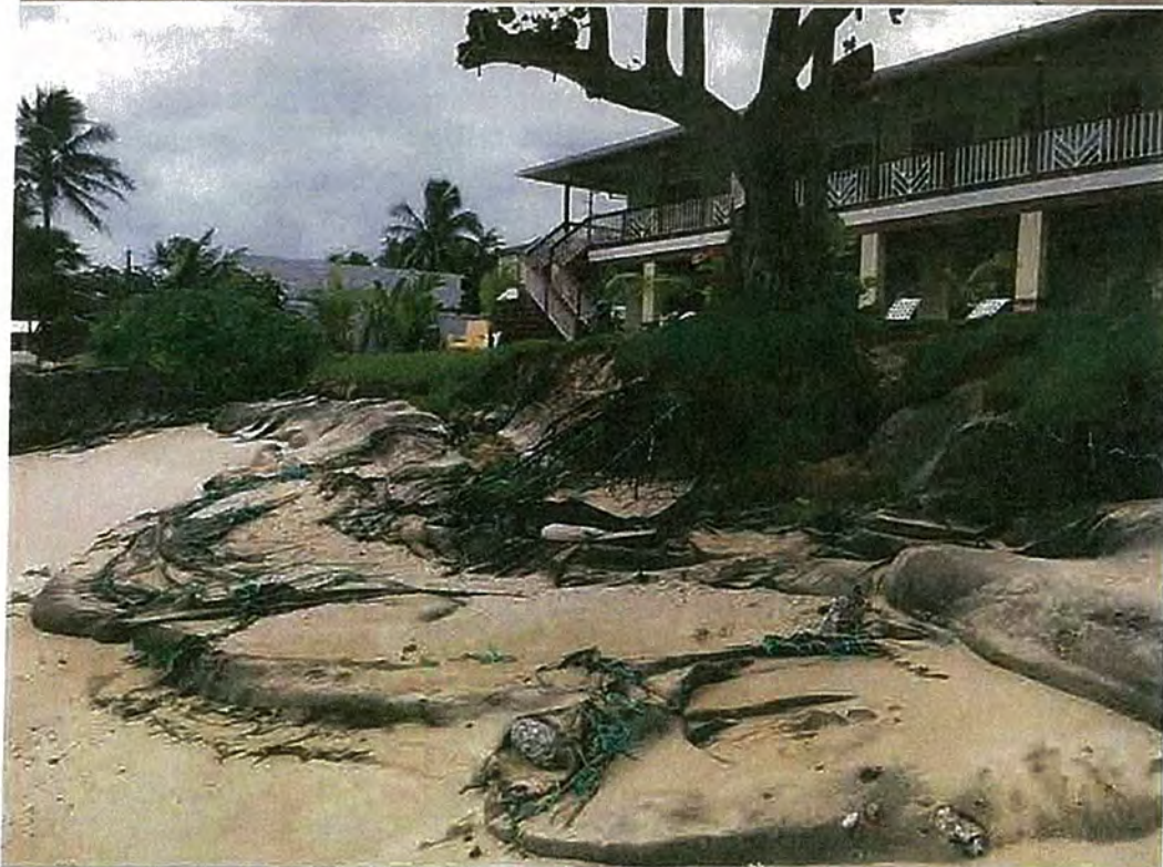
SEABags covered with black SEABlanket in disrepair
