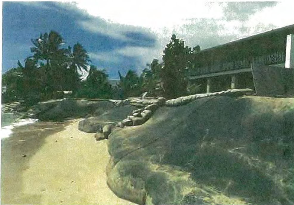
Completed Structure (Prchal) – View To South (NOTE: small sandbags and wooden rail to be removed)
