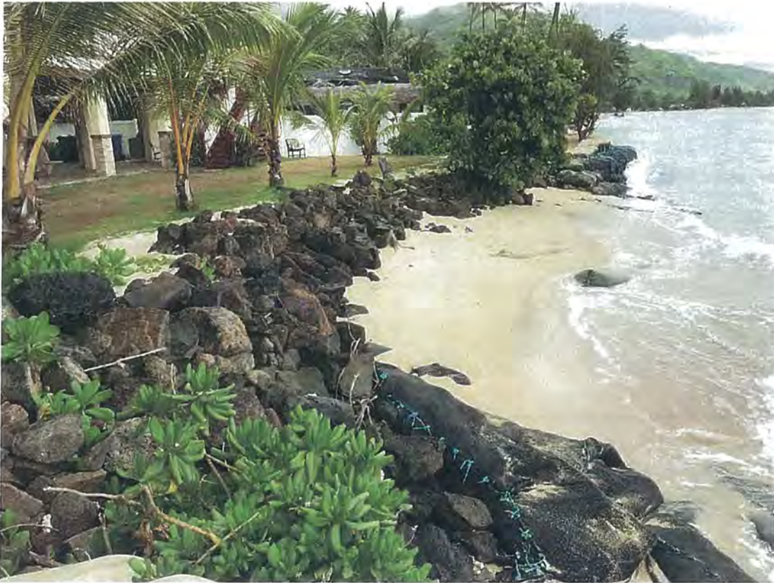
Figure 19: July 2, 2020 OCCL Photo of Alleged Unauthorized Rock Revetment & Erosion Control Materials
