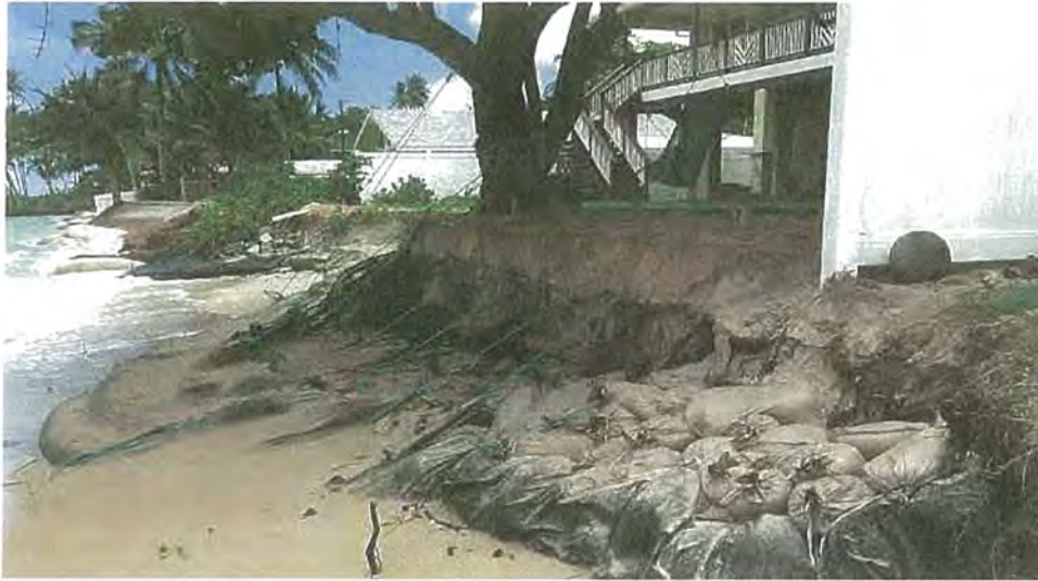
Figure 11: September 2014 Photo Showing Property's Current Residence & Failed Temporary Erosion Control Measures
