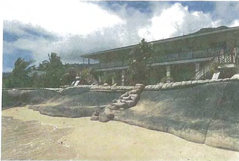
Completed Structure (Prchal) – View To South (NOTE: small sandbags and wooden rail to be removed)
