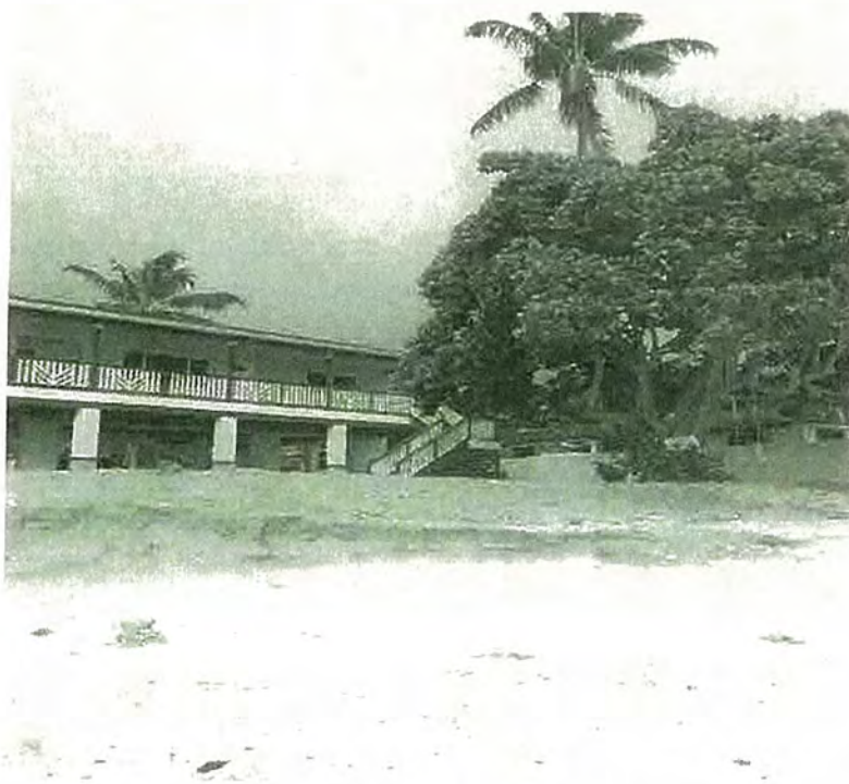
Fields erosion scarp at center of property July, 2014
