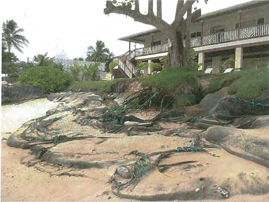
Figure 15: June 27, 2017 OCCL Photo Showing Property's Shoreline & Failed Temporary Erosion Control Structure
