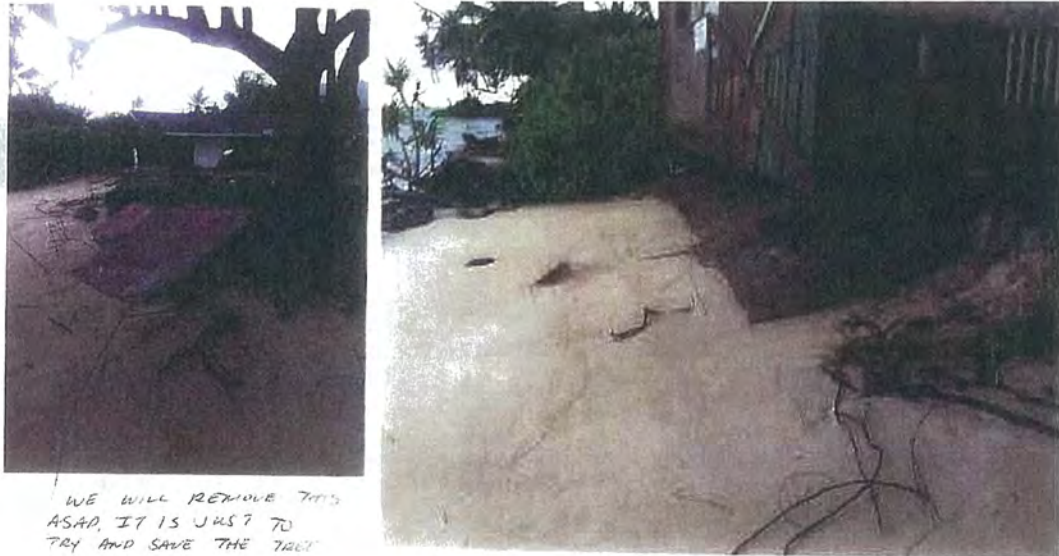
Figure 7: December 2012 Photo Showing Property's Previous Structure Being Threatened by Erosion
