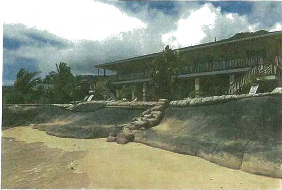
Completed Structure (Prchal) – View To South (NOTE: small sandbags and wooden rail to be removed)
