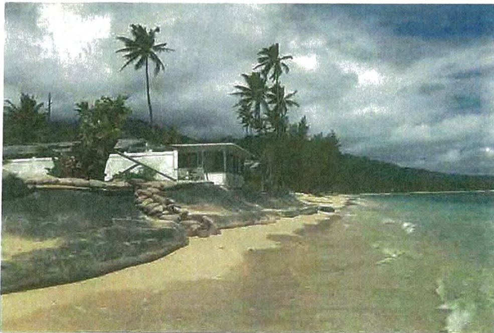
Completed Structure (Prchal) – View To North (NOTE: small sandbags and wooden rail to be removed)
