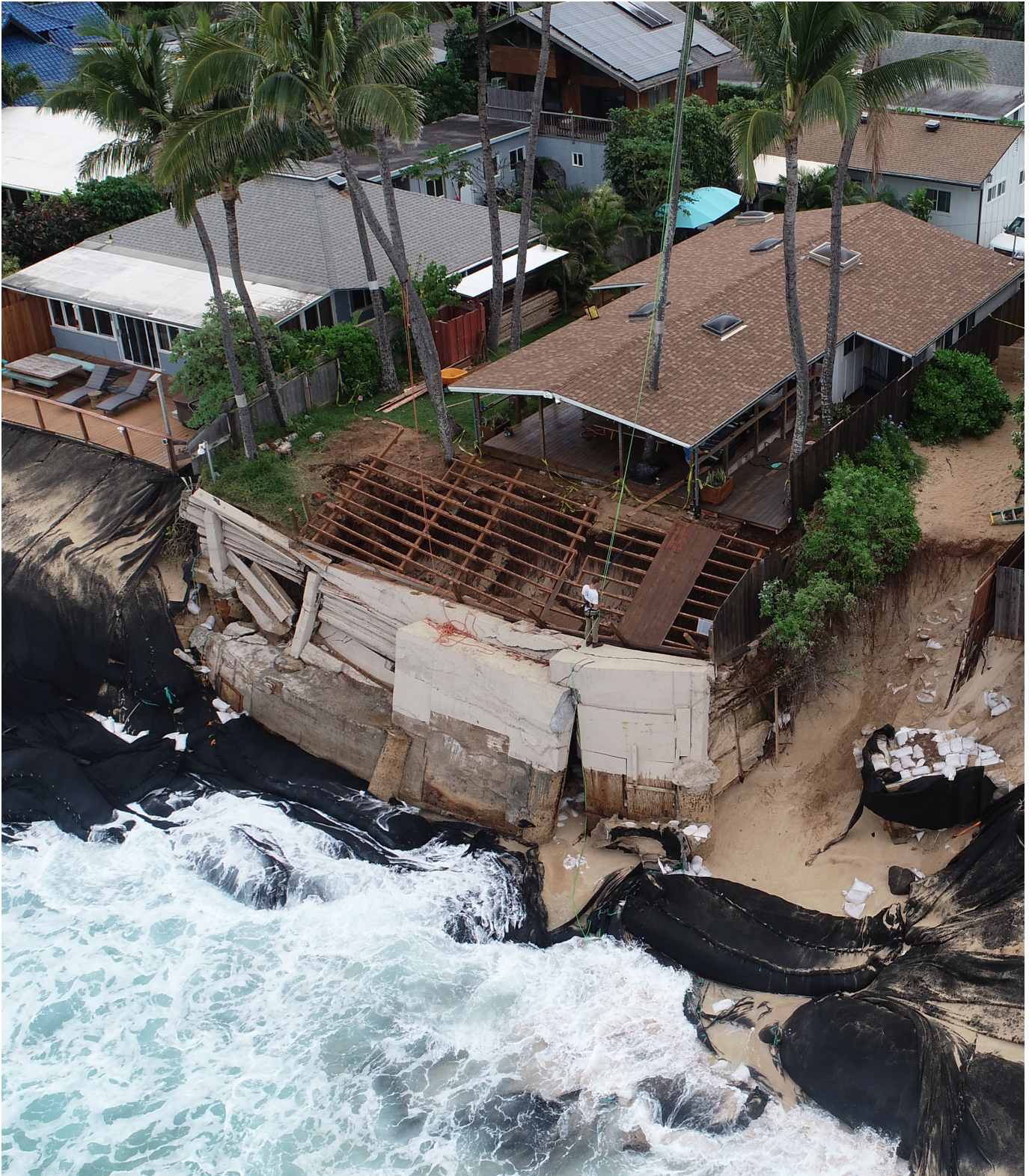
1/31/2022 OCCL Photo of Collapsed Seawall and other Unpermitted Shoreline Protection Devices in Shoreline Area Fronting the Subject Parcel
