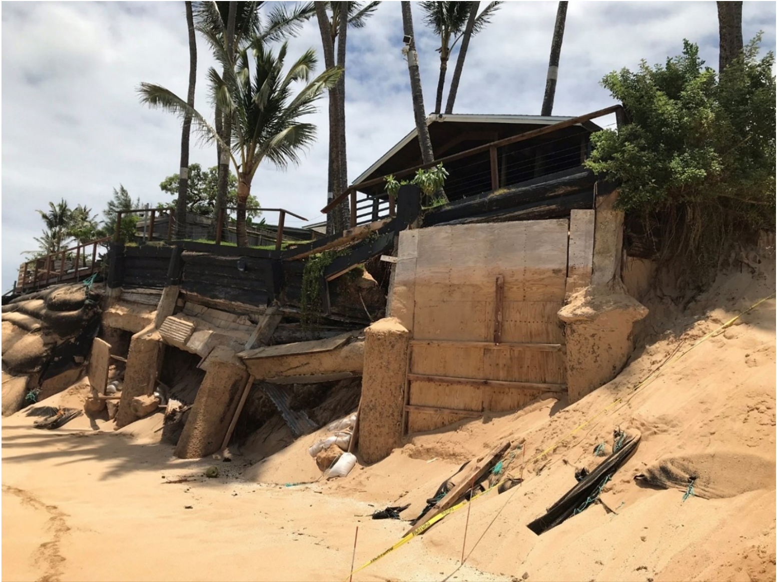
7/28/2020 OCCL Photo of Collapsed Seawall in Shoreline Area Fronting the Subject Parcel
