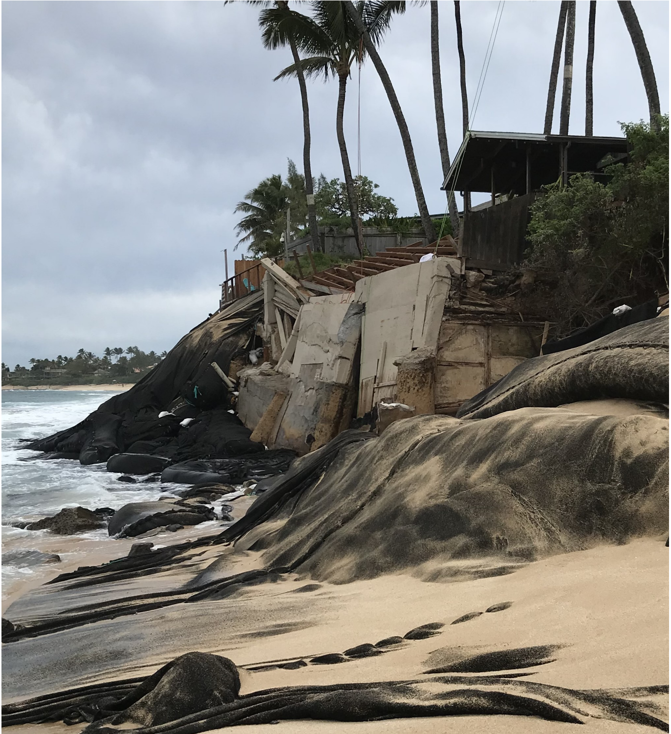
1/31/2022 OCCL Photo of Collapsed Seawall and other Unpermitted Shoreline Protection Devices in Shoreline Area Fronting the Subject Parcel
