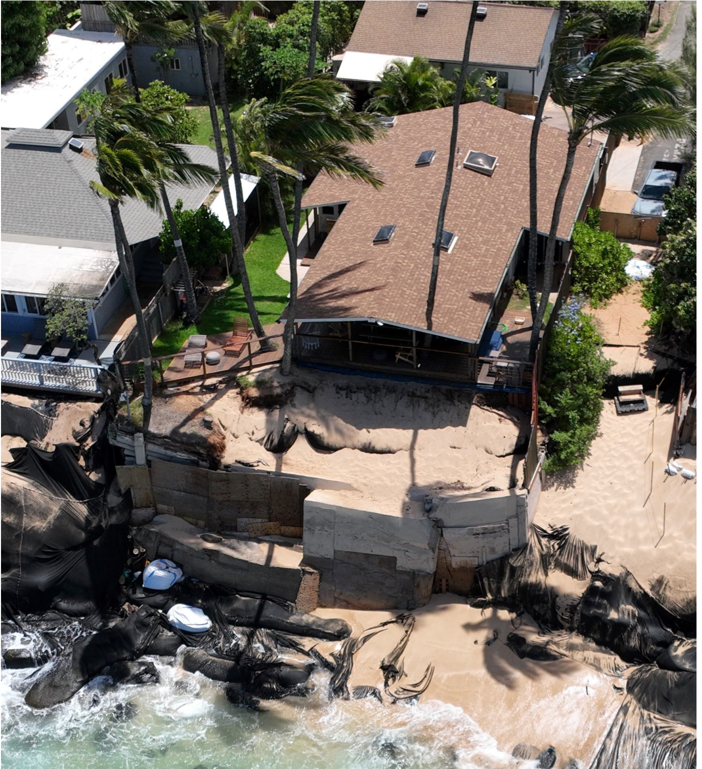
9/7/2022 OCCL Photo of Collapsed Seawall and other Unpermitted Shoreline Protection Devices in Shoreline Area Fronting the Subject Parcel
