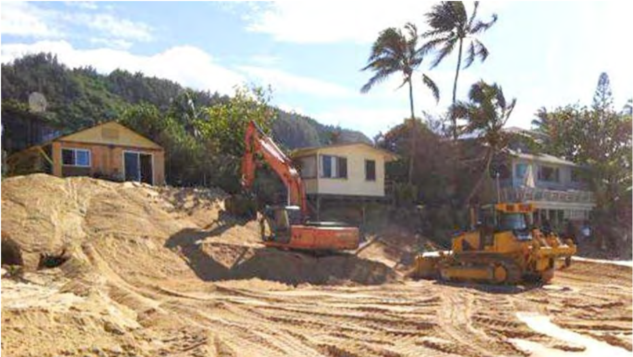
Excavator and Bulldozer doing 'Sand Pushing' on Sunset Beach (a couple houses away from McNamara)
