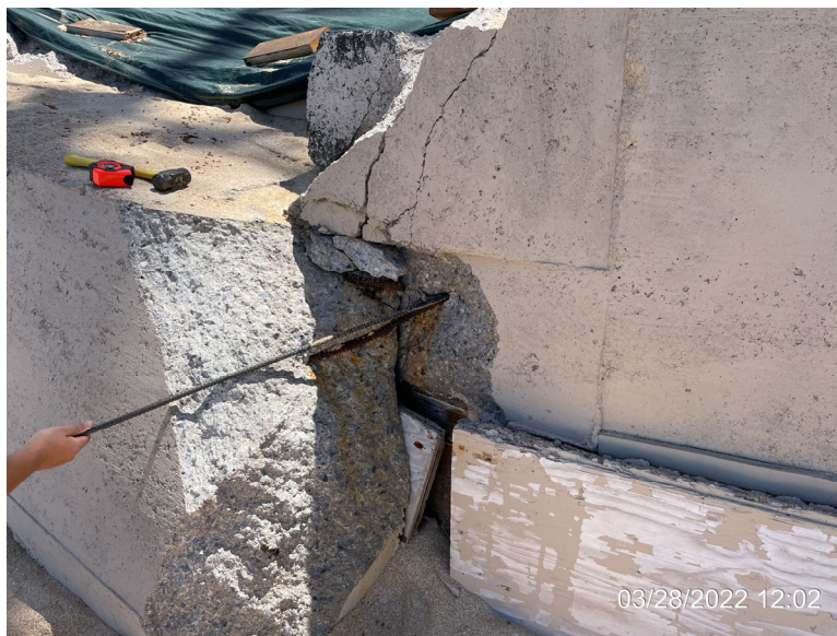
Photo 4: South side of property seawall facing mauka (showing broken concrete pieces, zoomed)
