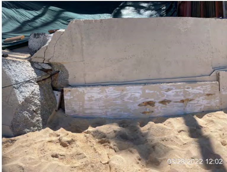
Photo 3: South side of property seawall facing mauka (showing broken concrete pieces)
