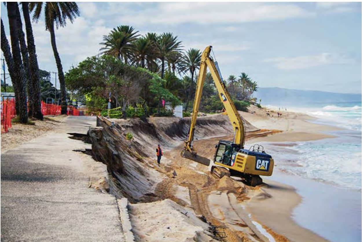
Excavator (in the wash of the waves) doing repairs associated with Sunset Beach Park Improvements 2018
