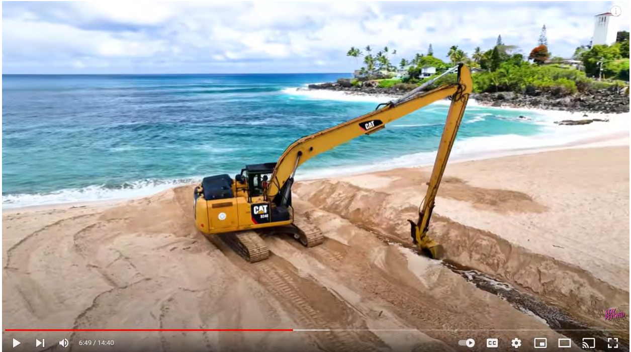
Excavator on Waimea Bay beach cutting channel to drain Waimea Valley River
