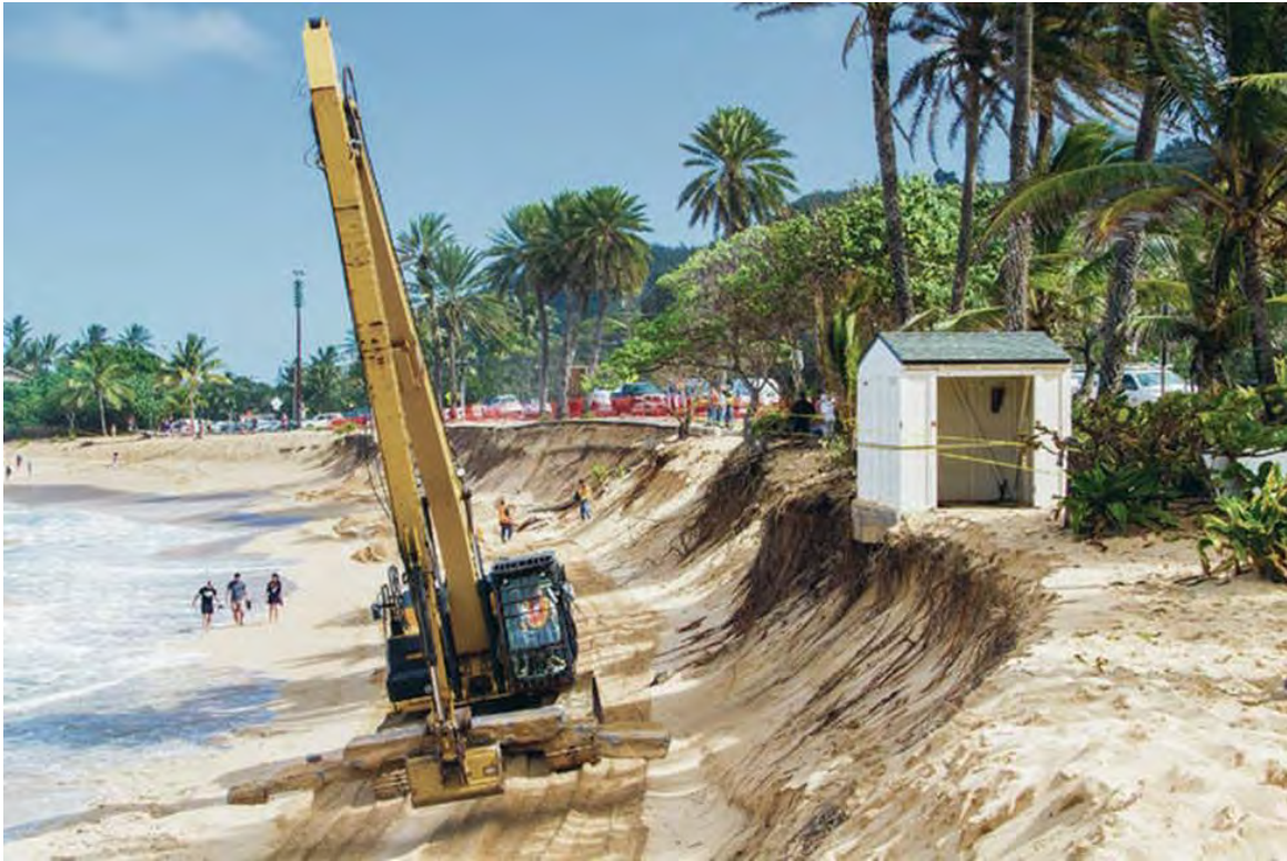
Excavator (in the wash of the waves) doing repairs associated with Sunset Beach Park Improvements 2018
