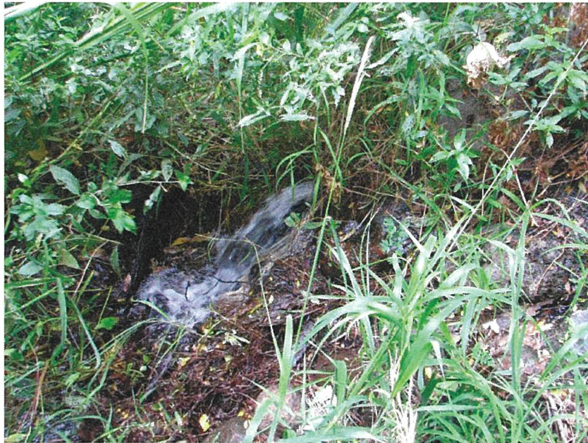
Figure 3. Seepage at the downstream face of Reservoir 3.
