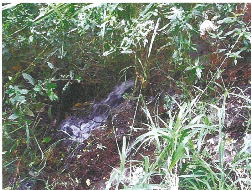
Figure 3. Seepage at the downstream face of Reservoir 3.
