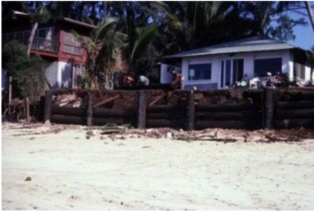
1977 Illegal seawall installation (brown house is Freemans)
