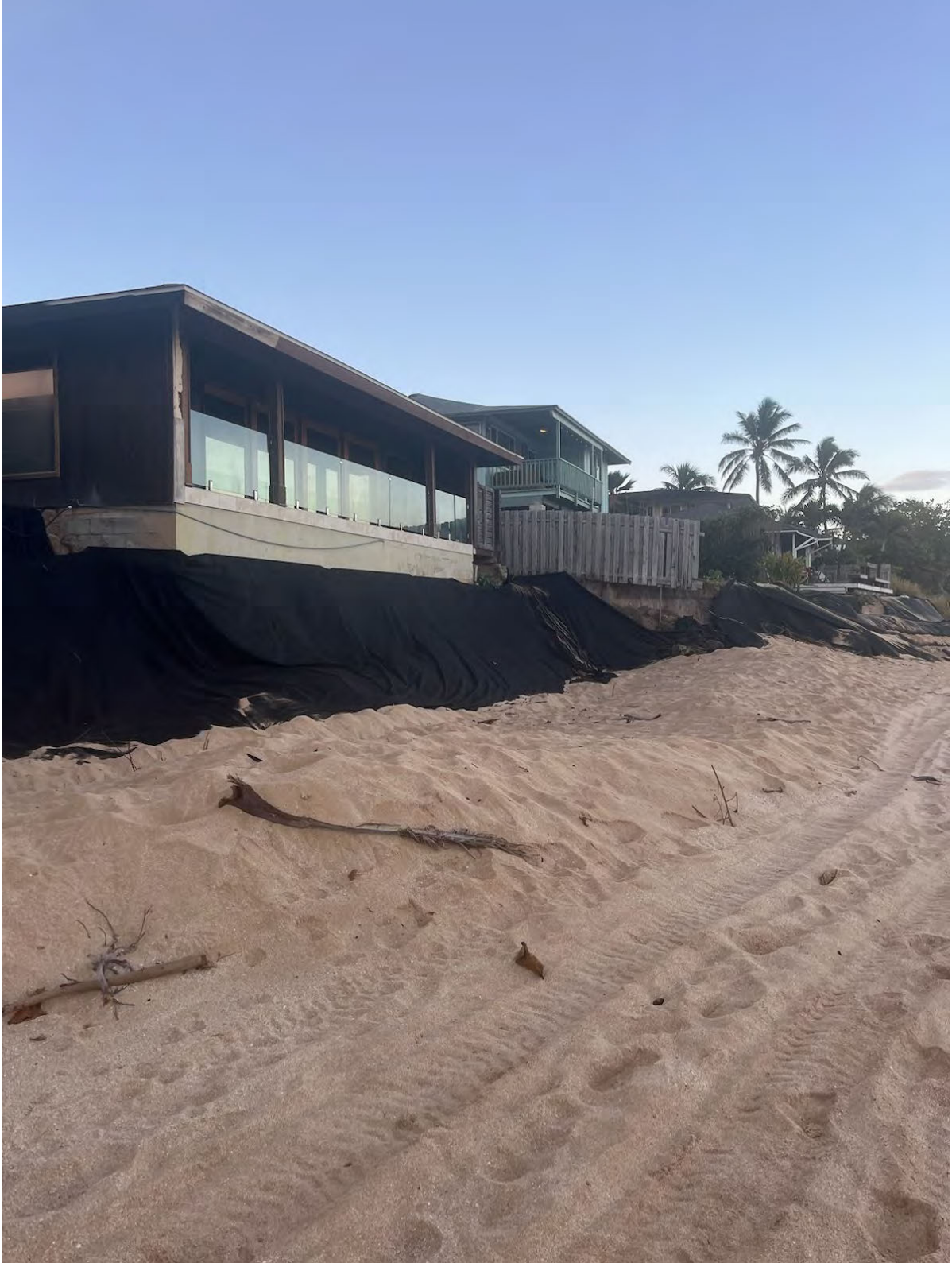
November 5, 2023 Additional Unauthorized Work in the Form of a Trench, Geotextile Tubes, and Geotextile Cloth
