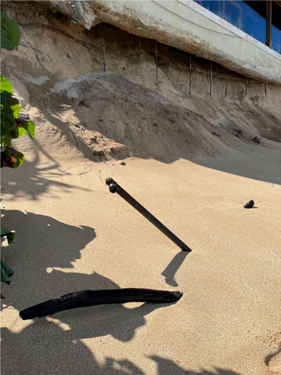
October 2, 2023 Remnant material from geotextile tubes found in sand
