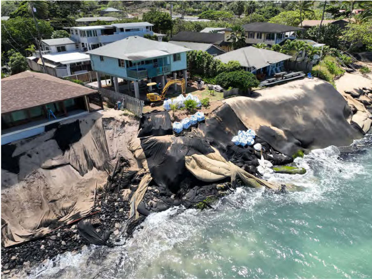
9/7/2022 OCCL-Photo of Mr. Youman and his Agent Installing Unauthorized Sandbags in the Expired and Unauthorized Erosion Control Structure in the Shoreline Area Fronting the Subject Parcel
