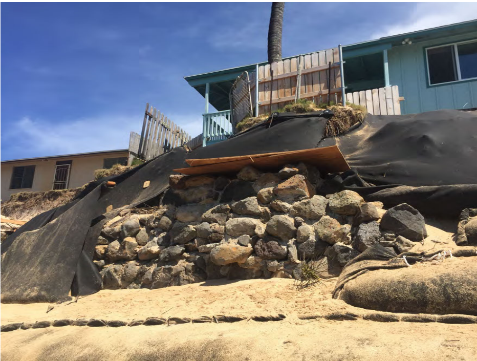
8/14/2018 OCCL Photo of Shoreline Area Fronting the Subject Parcel (Emergency CDUP OA 19-01); Debris/Unauthorized Materials (Failed Cement Wall) Being Utilized in the Temporary Erosion Control Structure
