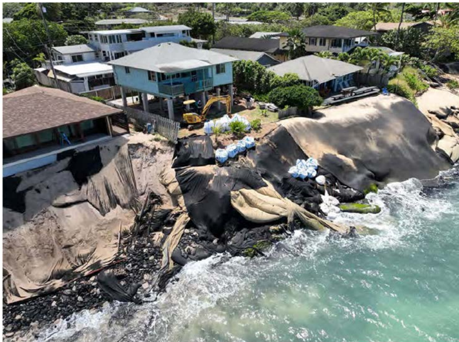
9/7/2022 OCCL-Photo of Mr. Youman and his Agent Installing Unauthorized Sandbags in the Expired and Unauthorized Erosion Control Structure in the Shoreline Area Fronting the Subject Parcel
