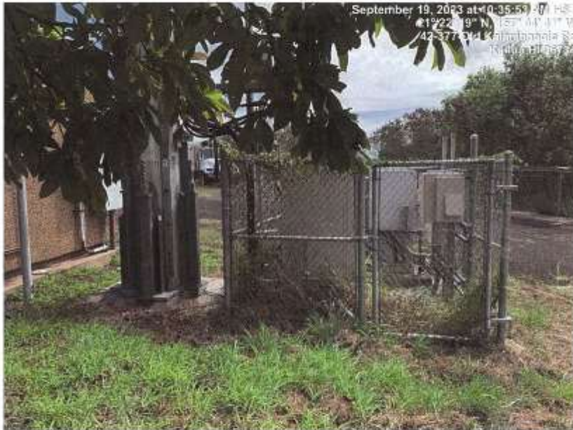
Figure 5: Easement D and Easement B (base of Antenna)
