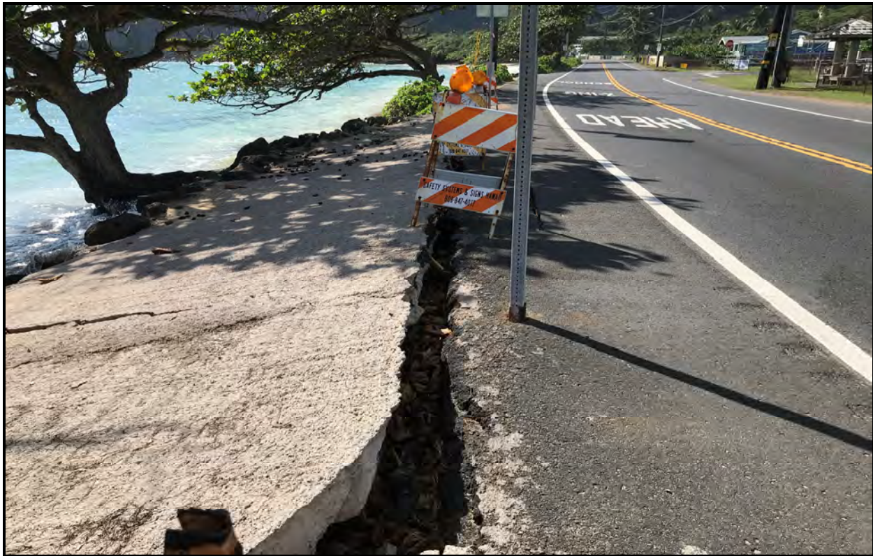
View of concrete cap separating from Kam Hwy road shoulder.
