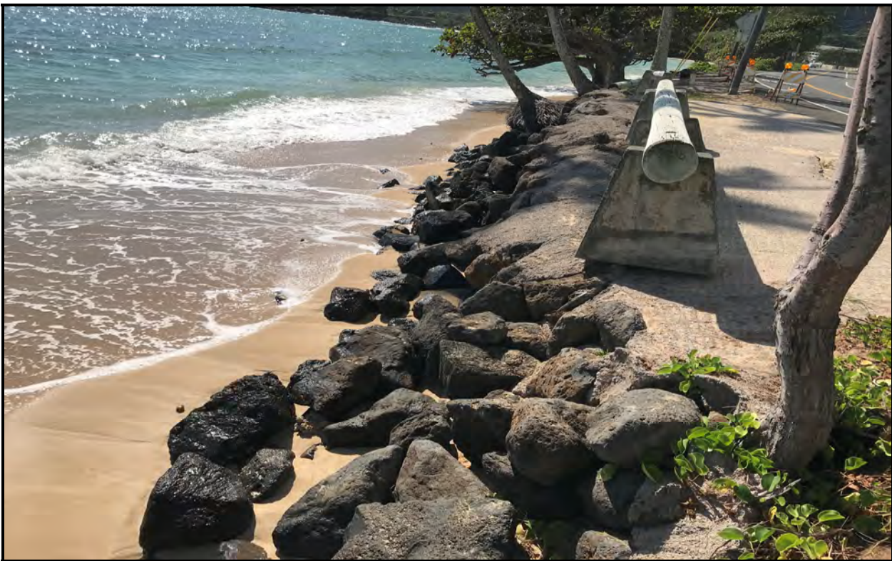
View of temporary revetment boulders being dislodged and narrowed Kaaawa beach.
