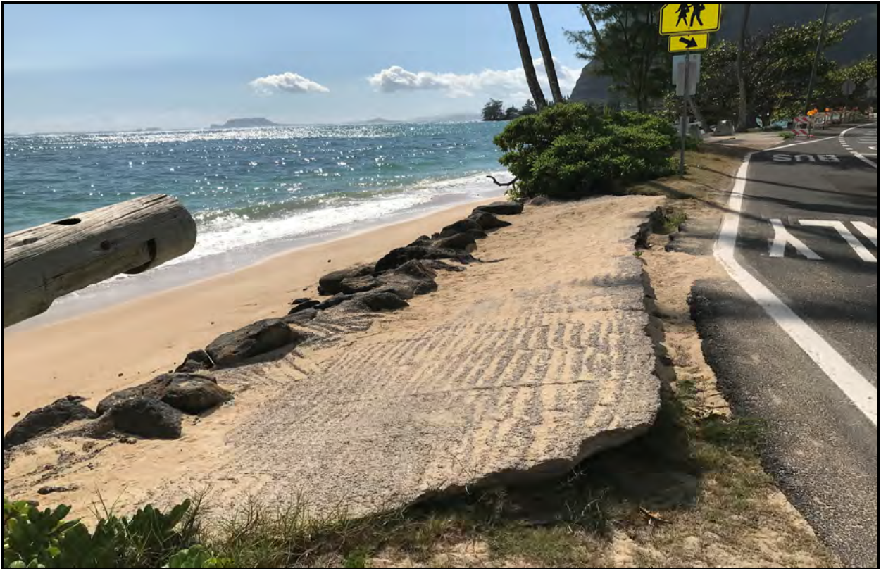
Temporary revetment and concrete cap separating from Kam Hwy road shoulder.
