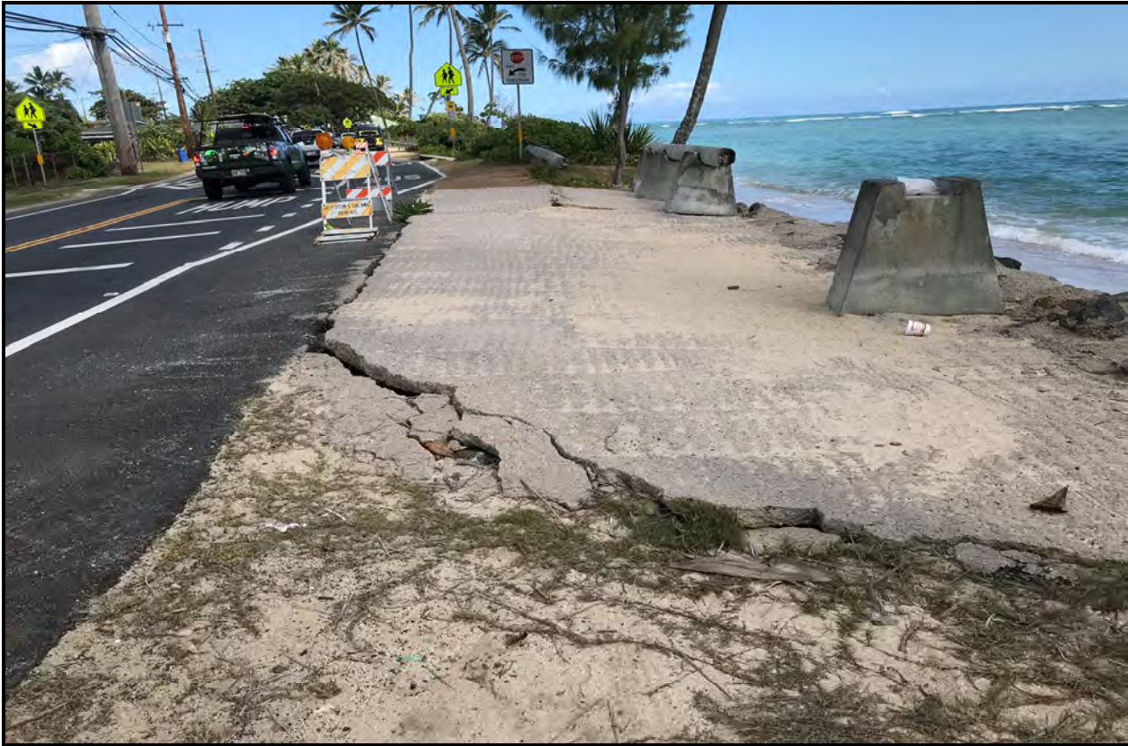
View of concrete cap separating from Kam Hwy road shoulder and safety barrier.
