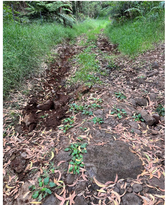
Figure 24. Roadways in KKCMA can get washed out and hard to pass due to erosion
