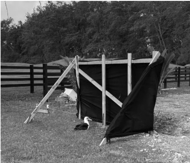
Figure 1. A wall of wood and shade cloth was erected while the Mōlī was incubating during unpermitted construction on Ms. Kan's property in December 2021.
