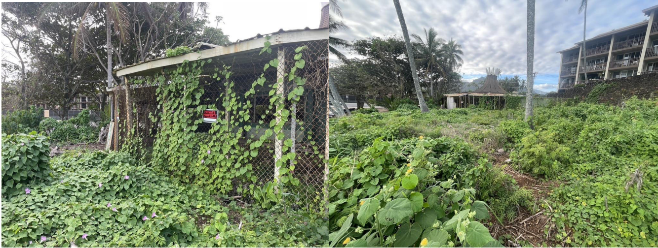
Images: View looking back at encroachments of old restaurant structure. Left picture shows roughly the section of the former restaurant structure that is encroaching onto the State parcel.
