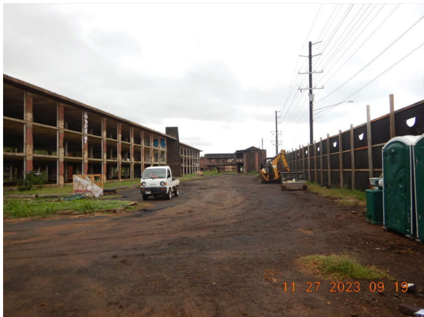
Photograph 14: View, facing north, of the road located between Building 1 and Kuhio Highway. Note the dust fence, heavy equipment, portable toilets, and handwashing station located in the enclosed area. Also, the road is covered with a layer of dirt, gravel and sand. The road is being used for vehicle and equipment to traverse the Site (see photograph 15). Photograph taken by Rande Tubal on November 27, 2023.
