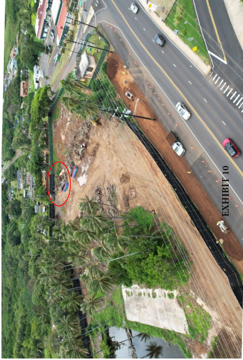
Image 5: Copy of "Exhibit 10" provided in RP21 Coco Palms' response to the NAV-RFI. This image depicts an aerial view of the cleared area and construction debris at the Site. Note that the actual area cleared of vegetation is greater than the area depicted in the Image 4 showing the trees intended for removal. Also note the piles of root balls (red circle), stockpiles of construction debris, exposed soils, and heavy equipment present at the site.
