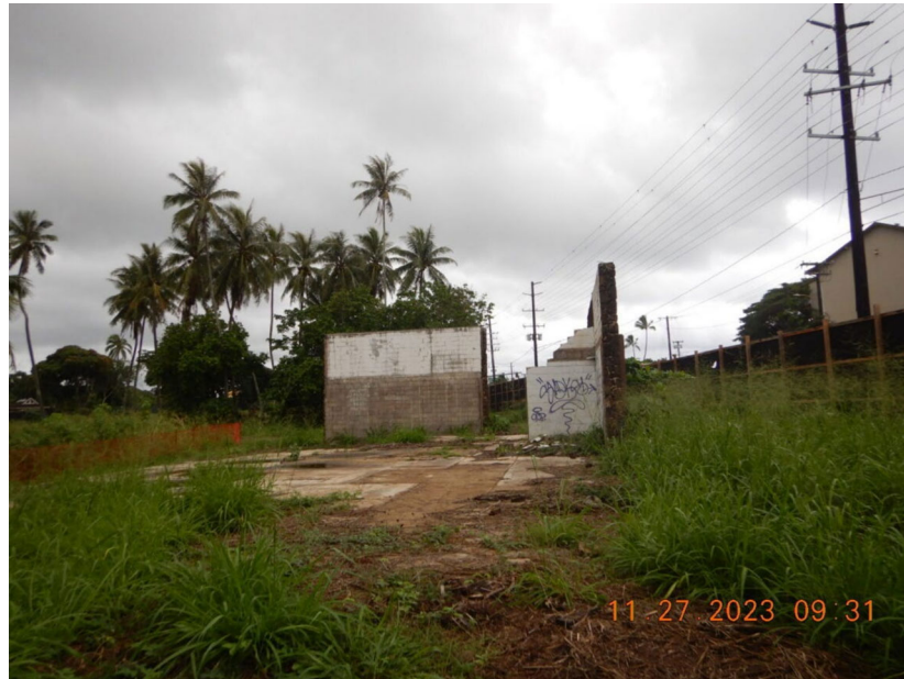
Photograph 21: View of the walls on Parcel 7, slated for demolition. Photograph taken by Rande Tubal on November 27, 2023.
