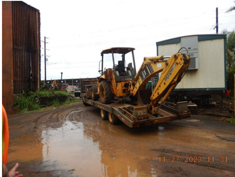
Photograph 15: View, facing northwest, of heavy equipment being trucked onto the Site. Photograph taken by Randee Tubal on November 27, 2023.
