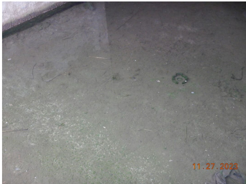
Photograph 8: Close up view of the standing water located in the underground parking structure beneath Building 1 (see Image 3). Photograph taken by Bobbie Teixeira on November 27, 2023.
