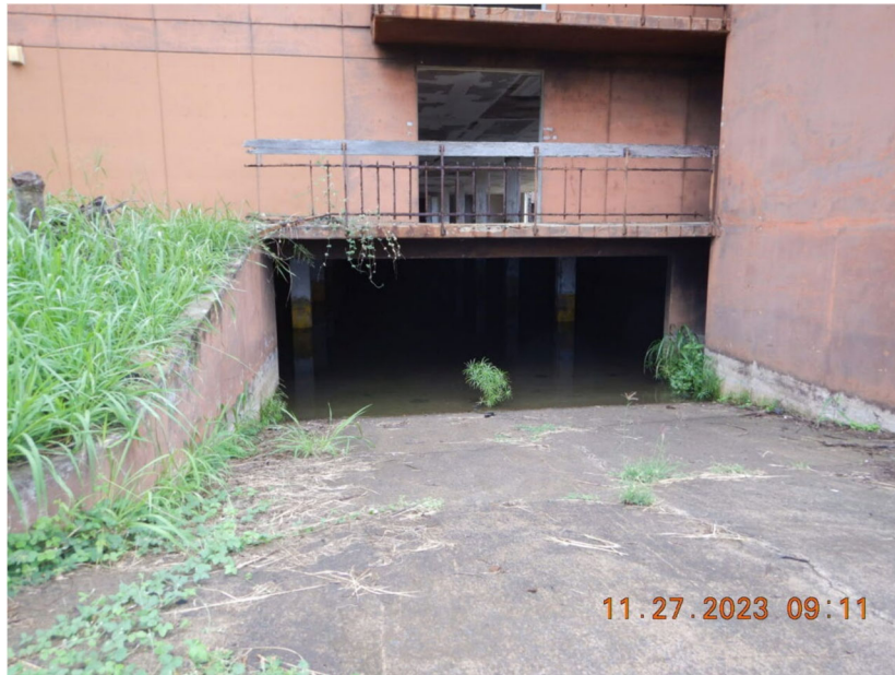
Photograph 7: View, facing north, of Building 1. Note the standing water located in the underground parking structure. Photograph taken by Randee Tubal on November 27, 2023.
