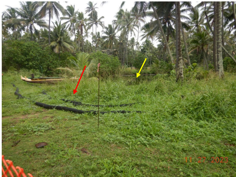
Photograph 18: View, facing northwest, of the southern end of the fishpond (yellow arrow). Note the double layer of filter socks placed around the fishpond (red arrow). Photograph taken by Bobbie Teixeira on November 27, 2023.
