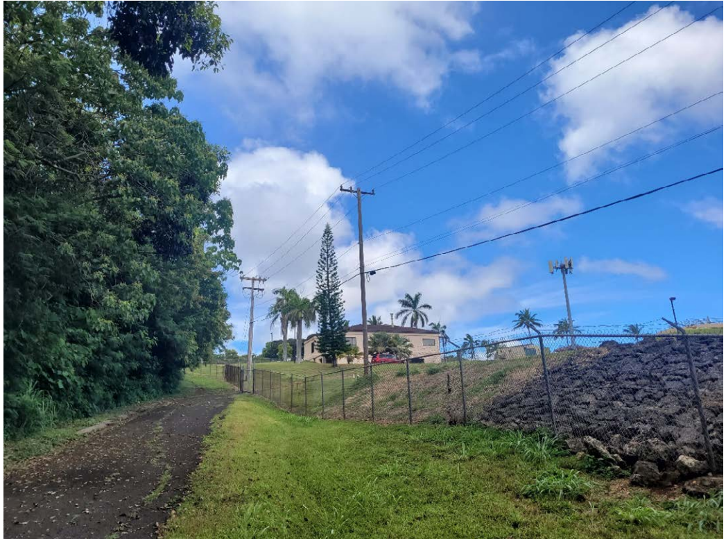
View of existing Hawaiian Electric power lines and poles in vicinity of proposed tap.
