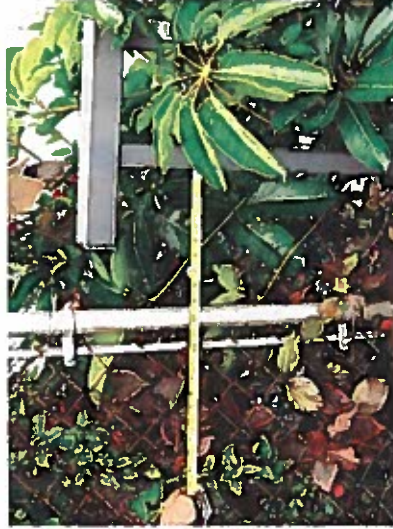
Depicts guardrail openings greater than 4 inches when walking surface is above 30 inches from the grade below at the pool area.
