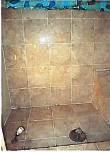
Photo of Room 210, Interior renovation performed with no record of Building Permit's. Newer Shower Unit.
