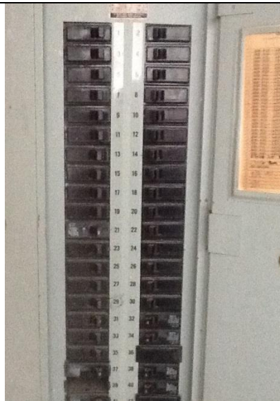
Guestroom corridors (All floors) Electrical room load centers require seals for unused openings.
