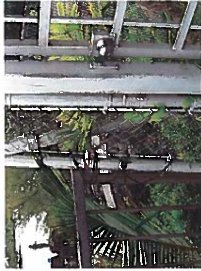
Depicts guardrail fasten to pool barrier with nylon rope.
