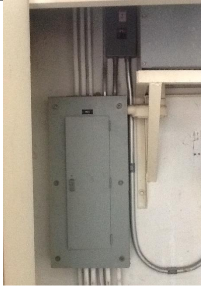
3 rd floor guestroom corridors electric room load center overcurrent protective devices too high 6'-7" max height
