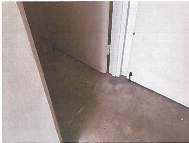
Self closing doors cannot be propped open, hardware not essential to door operation cannot be used
