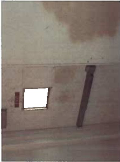
Depicts exit door at bottom of Makai stair enclosure. (illuminated exit sign required above or adjacent to the door)
