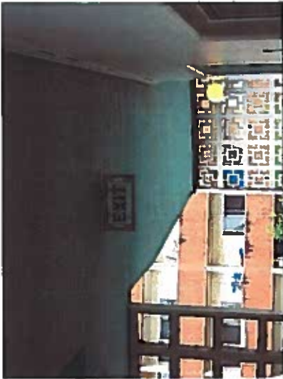
Depicts defective illuminated exit sign.
