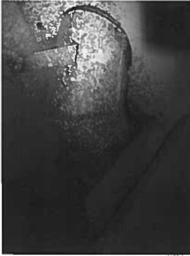
Depicts duct penetrating 1 hour corridor wall fire assembly. (annular space around duct not protected)
