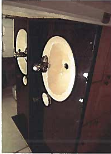
Photo of Room 210, Interior renovation performed with no record of Building Permit's. Newer Wash Basin.
