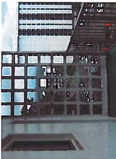
Depicts guardrail openings greater than 4 inches when walking surface is above 30 inches from the grade or roof below.
