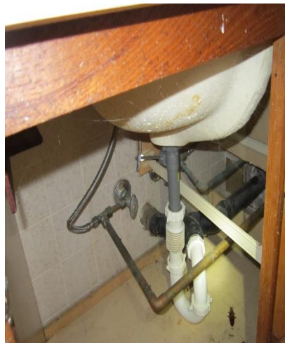
Up close photo of that wash basin where water and waste piping were installed to accommodate for kitchen sink
