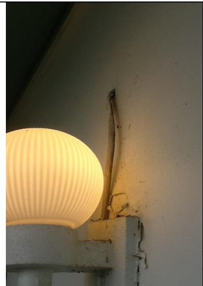
Guestroom corridors (All floors) Light fixtures above entry doors wired with NMB cable. Protection required.
