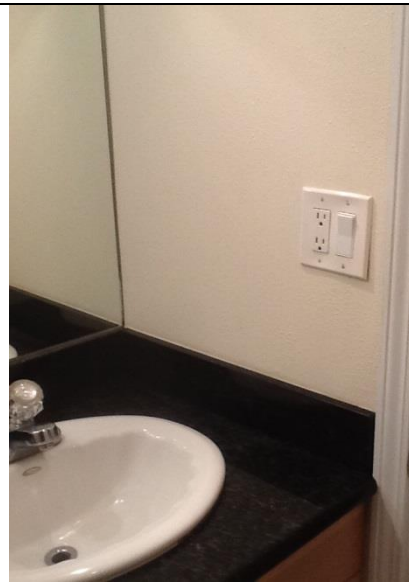
2 nd floor guest room 210 Receptacle next to bath sink GFCI protection required
