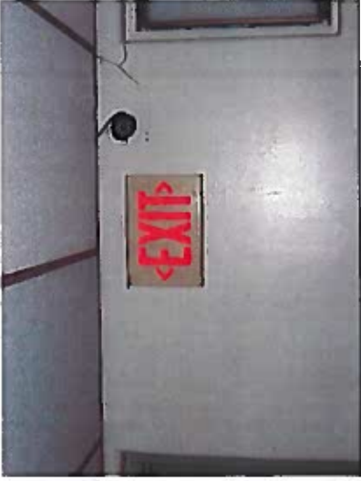
Depicts exit sign with two directional arrows on second floor. (one arrow points to an area with no exit)
