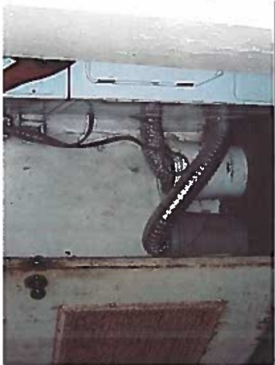
Depicts entry to machine room and dryer vents venting into a bucket.
