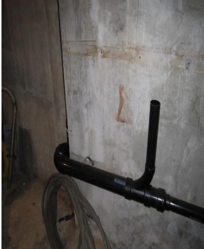
Installation of 4" x 2" ABS Combination Fitting, according to Maintenance Personal serves as an overflow point in the event of a wastewater back-up.
