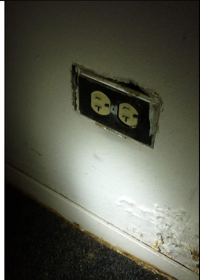
Guestroom corridors (All floors) Check receptacle covers to see if properly seated.
