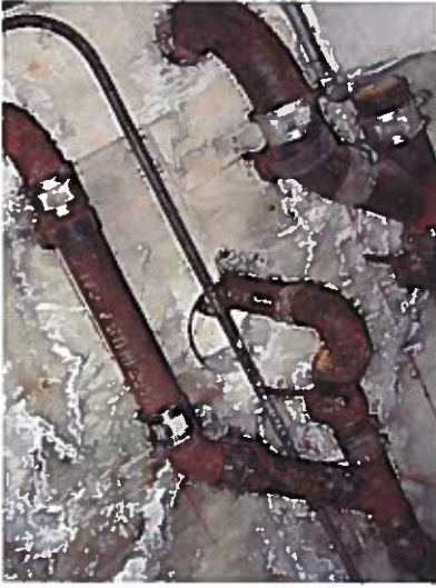
Depicts pipes penetrating 2 hour floor/ceiling fire assembly. (annular space around pipes not protected)
