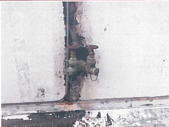
Please ensure all Fire Department Connections are in working order, as many are not in operational order at this time
