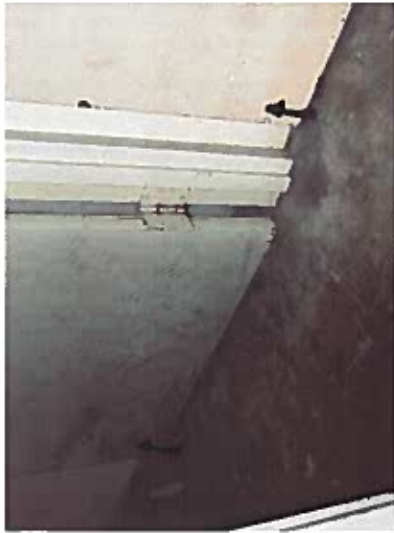
Depicts door stops used to keep exit door from self-closing.
