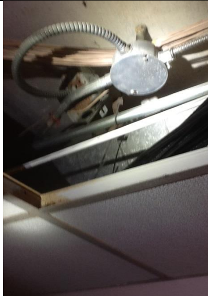
Guestroom corridors (All floors) junction boxes in ceilings covers required
