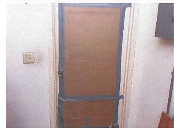
Remove cardboard from rated fire doors
