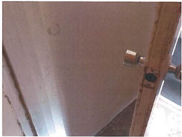
All hardware for doors shall be working and in good operational condition
