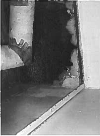
Depicts pipes penetrating 1 hour corridor wall fire assembly. (annular space around pipes not protected)
