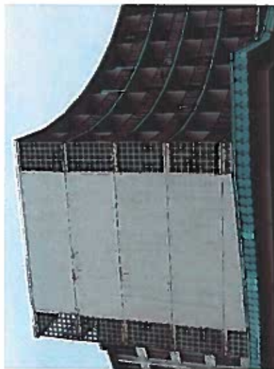
Depicts guardrail openings greater than 4 inches when walking surface is above 30 inches from the grade or roof below on the Mauka wing.
