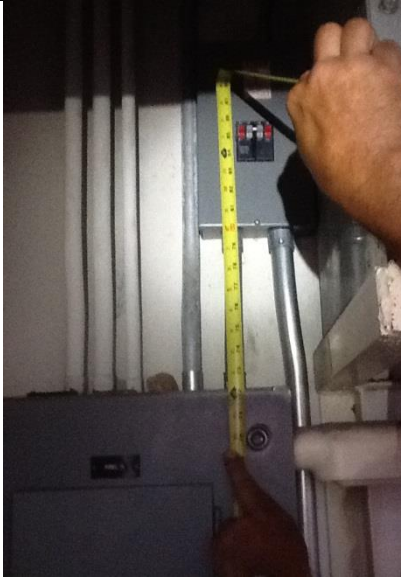
3 rd floor guestroom corridors electric room load center overcurrent protective devices too high 6'-7" max height. (7'-3") in field
