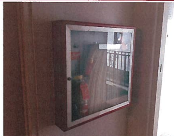
Fire extinguisher and hoses are not accessible, as glass does not have tool to break glass available
