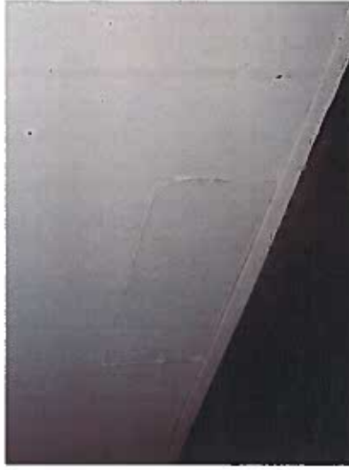
Depicts opening in corridor wall from unit 608. (fire tape or drywall tape around opening required)
