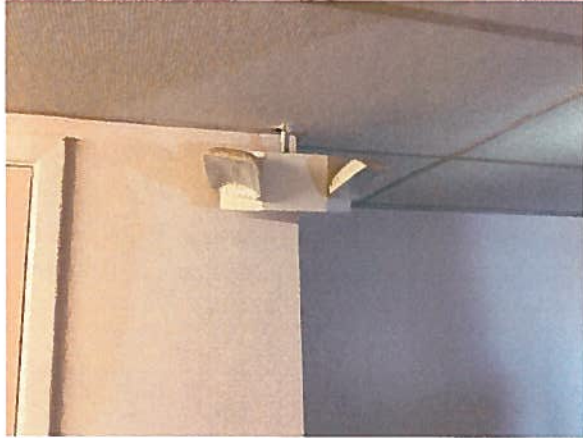
Please ensure all emergency lighting is fully operational
