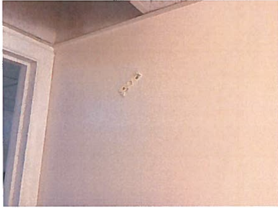
No smoke detectors in guest rooms as required by code
