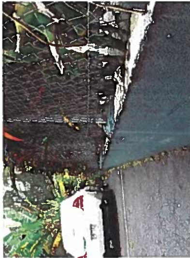
Depicts opening in pool barrier greater than 4 inches.
