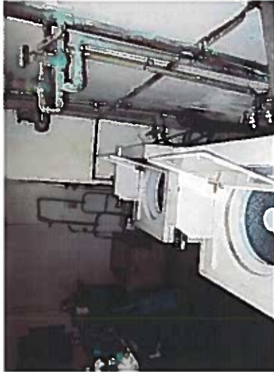
Another photo of Hotel Laundry Room.
