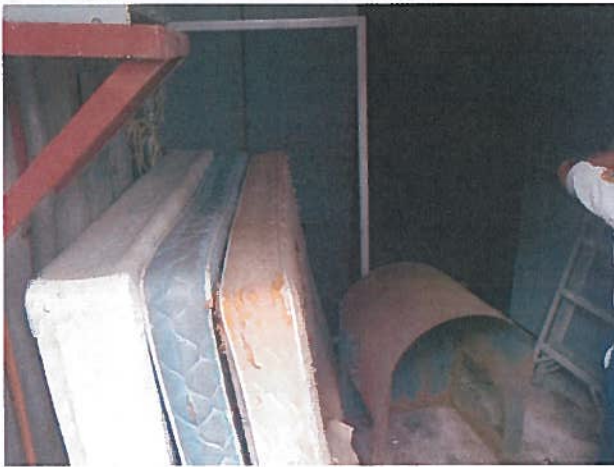
Remove combustibles from main electrical room, such as beds, and other flammables
