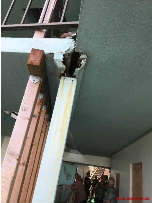
Photo 1) Depicts old walkway support and added 2 nd floor support.
