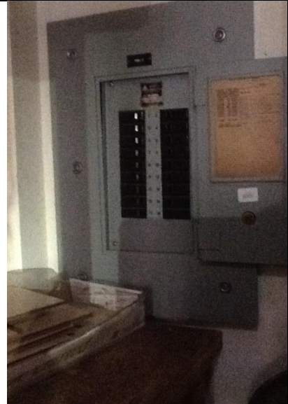
Storage rooms (all floors) Work clearance in front of this electrical panel required.
