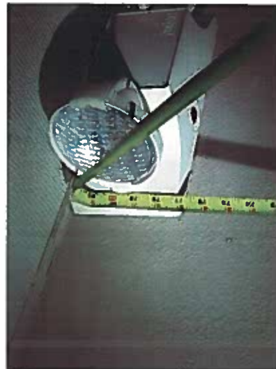
Depicts emergency exit lighting installed below 80 inches. (a barrier shall be provided were the vertical clearance is less than 80 inches)
