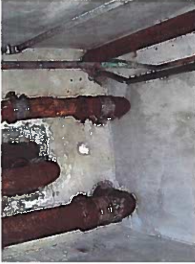
Depicts pipes penetrating 2 hour floor/ceiling fire assembly. (annular space around pipes not protected)
