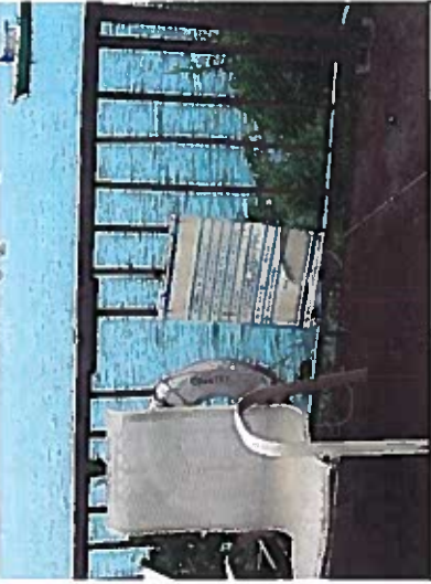
Depicts guardrail openings greater than 4 inches when walking surface is above 30 inches from the grade below at the pool area.
