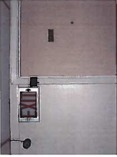
Depicts non-illuminated exit sign on the 5th floor.
