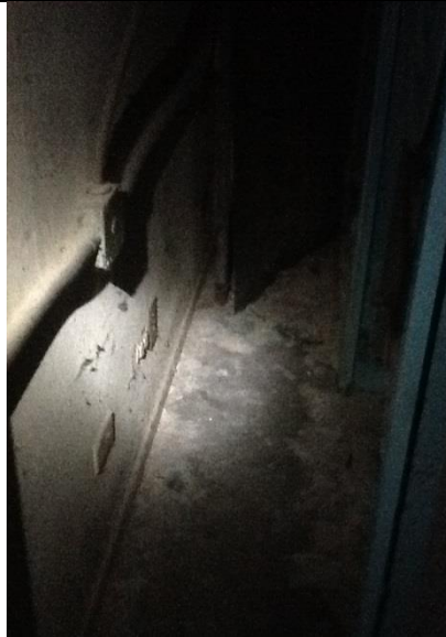
2 nd floor housekeeping room 209 Receptacle behind dryer missing faceplate.
