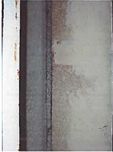
Depicts top of corridor wall on the 6 th floor. (Continuity of wall must go to the floor or ceiling above)
