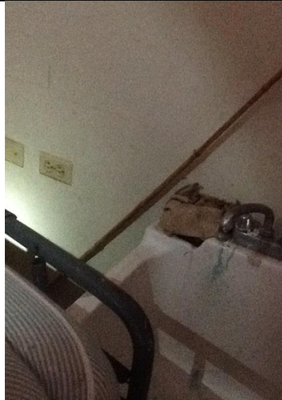
Storage rooms (all floors) Receptacles next to wash tubs require GFCI protection.
