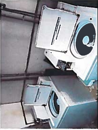
Photo of Hotel Laundry Room.
