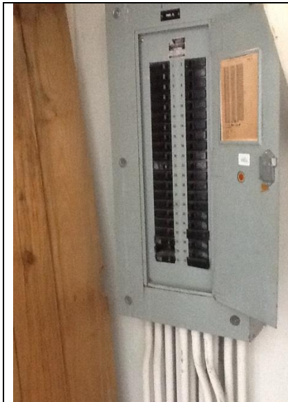
Guestroom corridors (All floors) Electrical room load centers require seals for unused openings.
