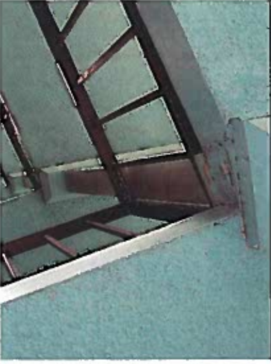
Depicts deteriorating concrete walkway supported by wood structural members. (wood material used in type IB construction must be heavy timber and have a fire-resistance rating of 2 hours)
