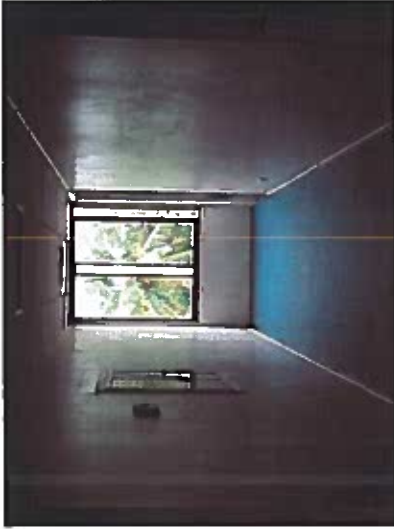
Depicts widow openings greater than 4 inches and the grade below is over 72 inches from the bottom of the opening.
