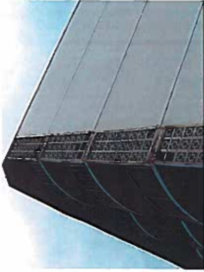
Depicts dilapidated screen tile at the rear of County Club.
