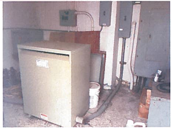
Please remove combustible storage from transformer room
