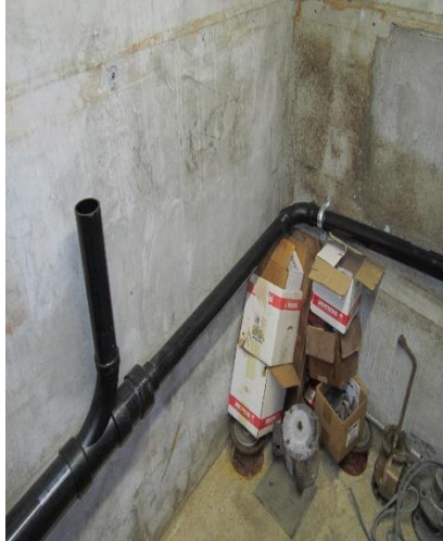
Another angle of that 4" ABS Pipe rough-in, 2" ABS Pipe receiving wastewater from Washer Machine Standpipe.
