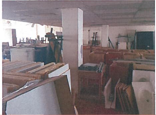
Banquet room: Doors are not to code, storage needs to be removed, doors on ocean side need to be unblocked
