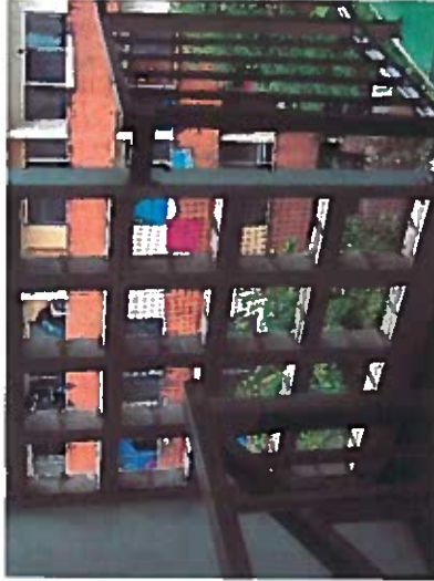
Depicts guardrail openings greater than 4 inches when walking surface is above 30 inches from the grade or roof below.
