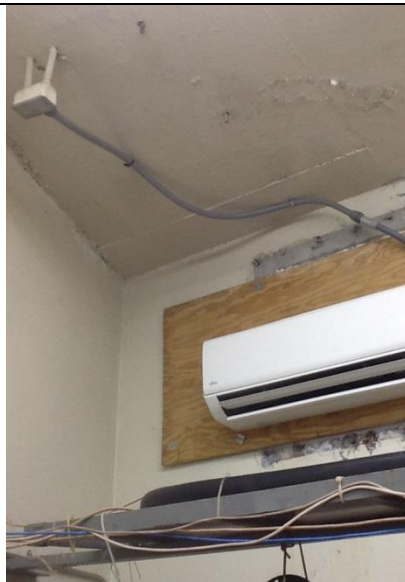
2 nd floor data/com room work AC unit disconnecting means required. Unsupported flexible conduit.
