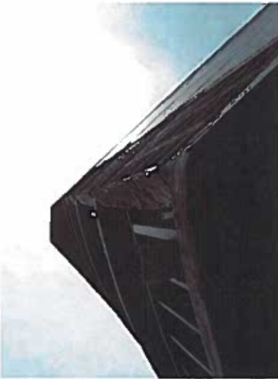
Depicts close up of dilapidated screen tile at the rear of County Club.
