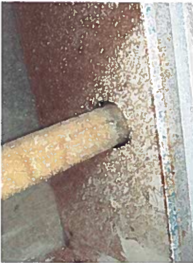
Depicts pipes penetrating 1 hour corridor wall fire assembly. (annular space around pipes not protected)
