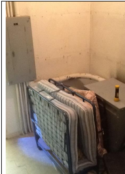
2 nd floor data/com room work clearance in front of electrical equipment.
