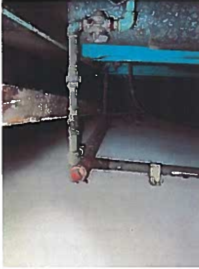
Photo of Gas Piping for Gas Dryer, in Hotel Laundry Room.
