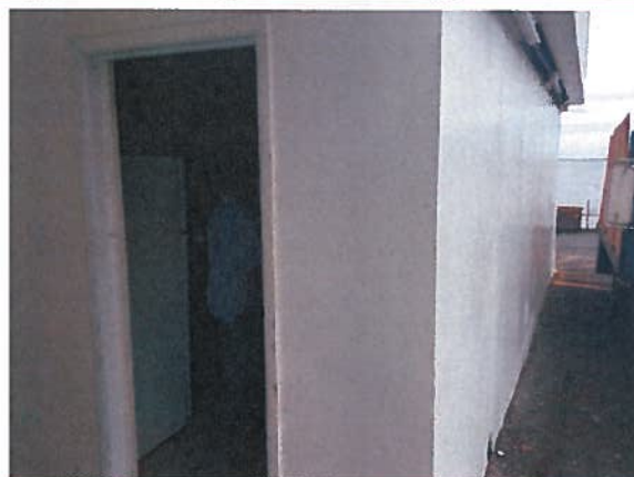
Storage on bottom has non Fire rated door, which may not be able to protect room and contents
