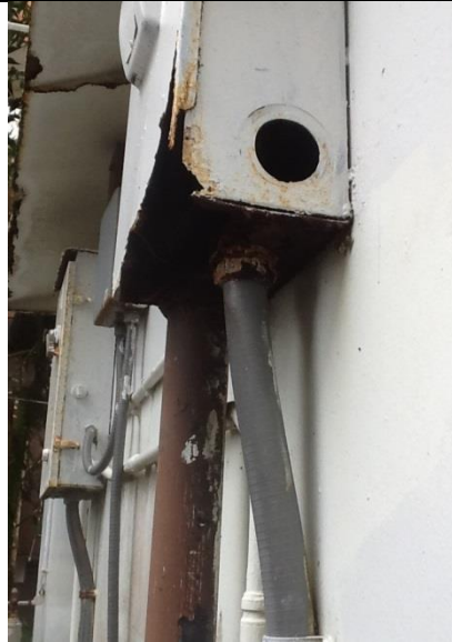
Exterior electrical equipment behind former restaurant deteriorated by means of corrosion. Required to be upgrade
