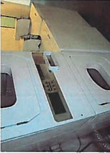
2 nd Photo of Laundry Area located on ground floor ocean side of building next to elevator.
