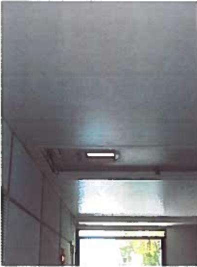
Depicts exit door. (illuminated exit sign above or adjacent to exit door required)
