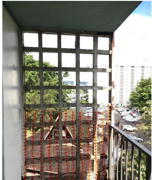
Photo 4) Depicts end wall partition on each floor with large openings present fall concerns.
