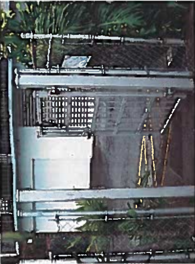
Depicts gate to pool area not closed. (gate should be self-closing and self-latching. Release mechanism located below 54 inches)
