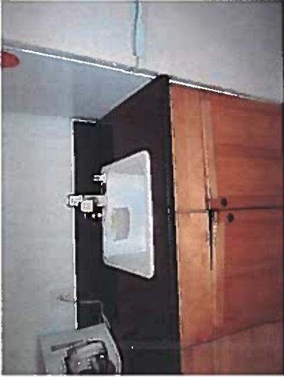
Photo of Room 210, Interior renovation performed with no record of Building Permit's. Newer Bar Sink.
