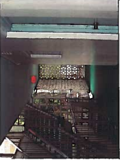
Depicts open exit stairway. (all openings, windows and doors, within 10 feet of an exterior exit stairway shall be protected)
