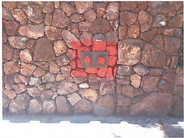
Fire Department connection does not have signage or annual inspection tag
