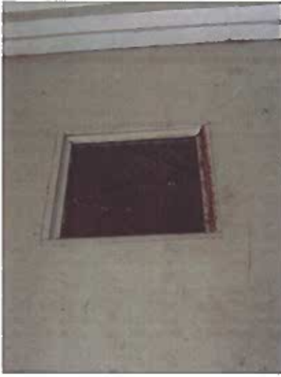
Depicts defective wired glass in a fire-rated door.
