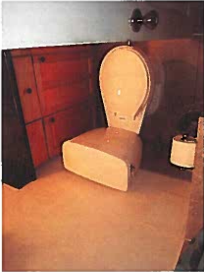
Photo of Room 210, Interior renovation performed with no record of Building Permit's. Newer Water Closet/Toilet.
