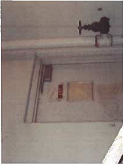
Depicts exit door at bottom of Makai stair enclosure. (illuminated exit sign required above or adjacent to the door)
