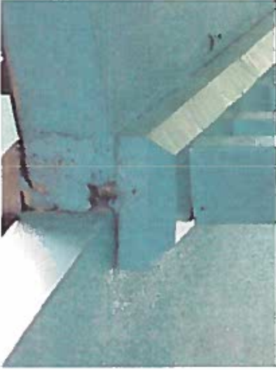
Depicts deteriorating concrete walkway supported by wood structural members. (wood material used in type IB construction must be heavy timber and have a fire-resistance rating of 2 hours)
