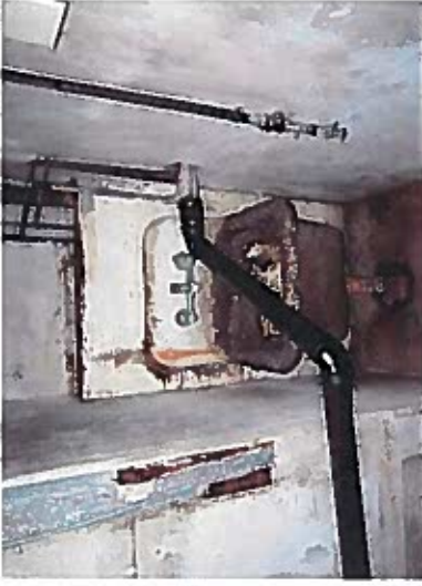
Photo of inside of Machinery/Equipment room, showing Plumbing pipe that has been installed for Laundry Area next to elevator.
