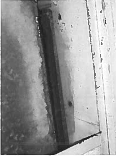
Depicts duct penetrating 1 hour corridor wall fire assembly. (fire/smoke damper required, annular space around duct not protected)
