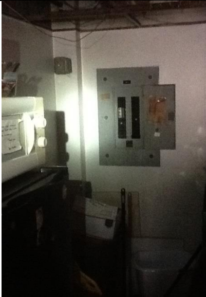
2 nd floor housekeeping room 209 work clearance in front of this electrical panel required.
