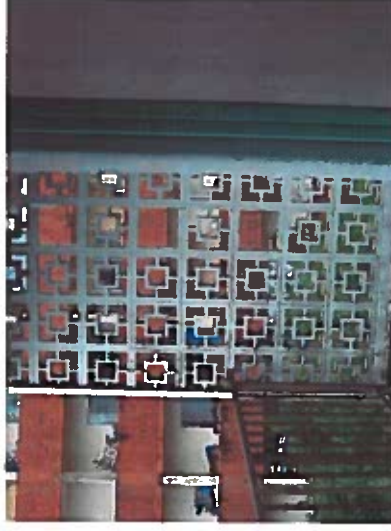
Depicts guardrail openings greater than 4 inches when walking surface is above 30 inches from the grade or roof below.
