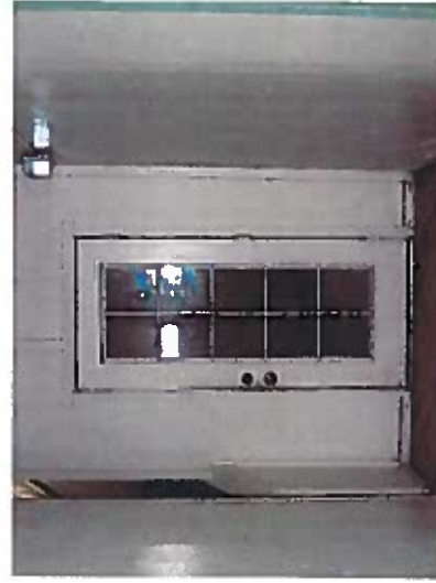
Depicts unpermitted room adjacent to the Mauka stairway on the ground floor.
