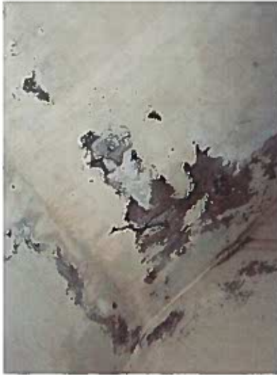
Depicts concrete spalling in the interior of the rear exit stairs.
