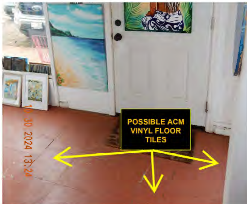
Figure 57. Possible ACM vinyl floor tiles (DSCN3994 Close Up).
