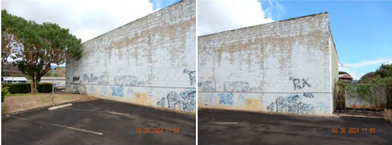
Figures 20 & Figure 21. Existing west / south-west CMU wall of auto repair shop with faded paint and graffiti (DSCN3699 & DSCN3700).
