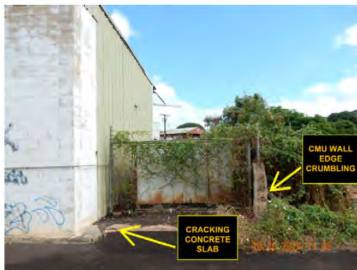
Figure 22. Locations of cracked concrete slab and crumbling CMU wall (DSCN3701).
