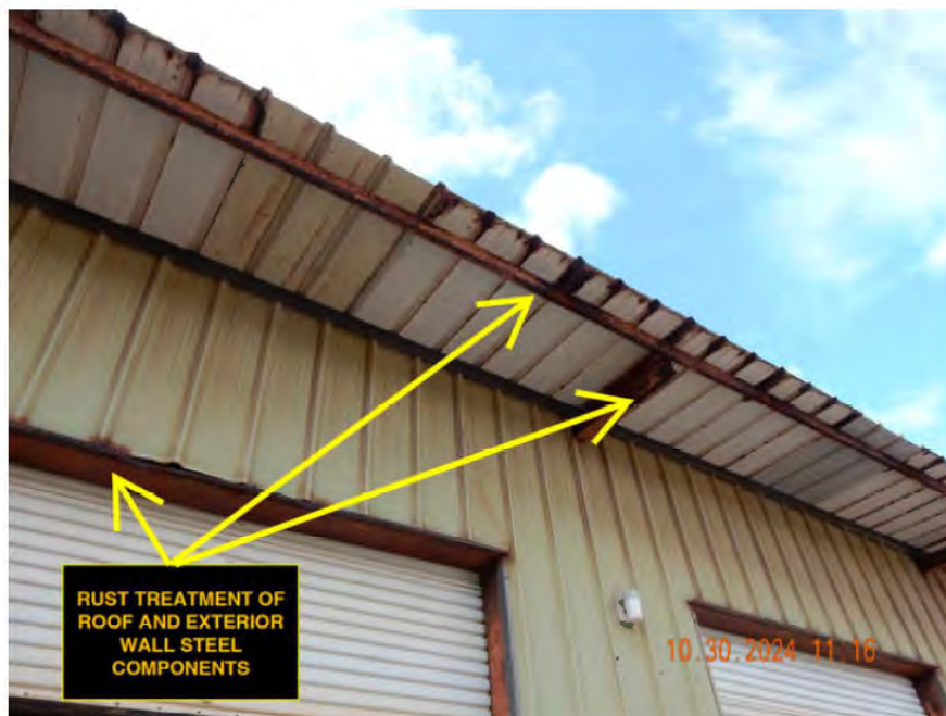
Figure 67. Rusting roof and exterior wall steel components (DSCN3757).
