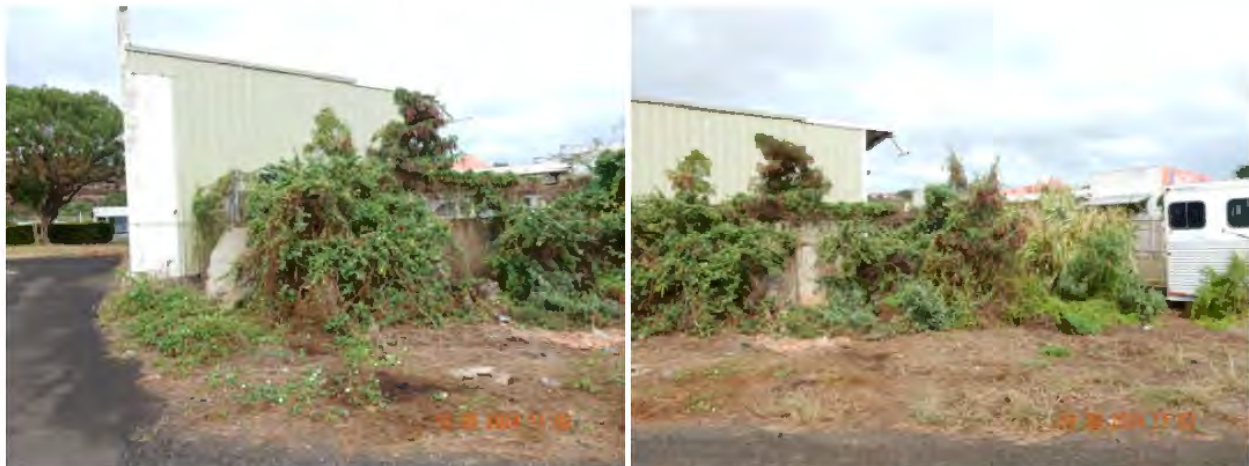
Figures 24 & 25. Overgrown landscaping (DSCN3703 & DSCN3704).
