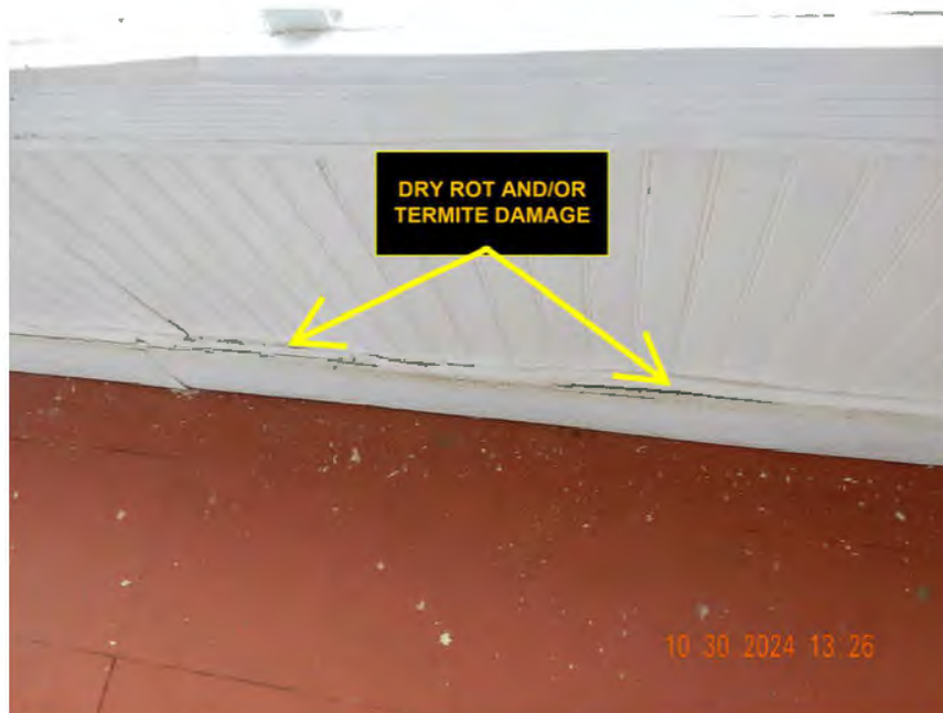
Figure 60. Dry rot and/or termite damage (DSCN4010).
