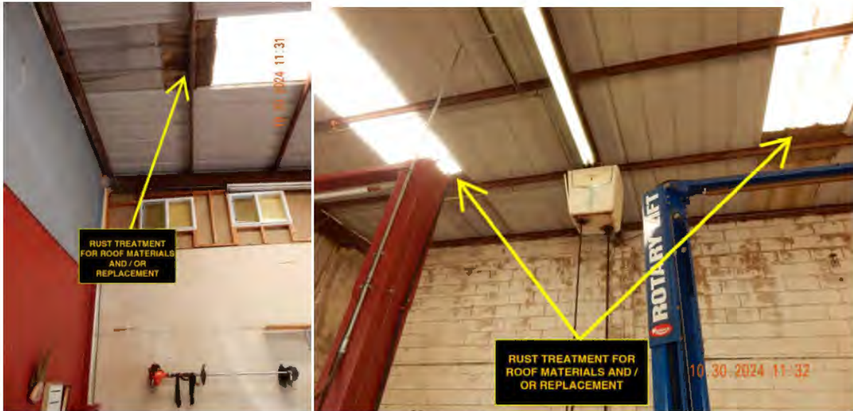
Figure 73 & 74. Rusted roof panels (DSCN3815 & DSCN3824).
