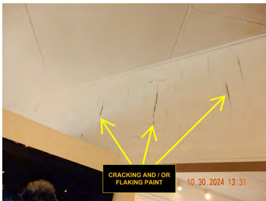
Figure 63. Cracking and / or flaking interior paint (DSCN4041).
