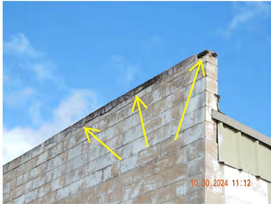
Figure 66. Cracked and crumbling CMU wall top (DSCN3735).
