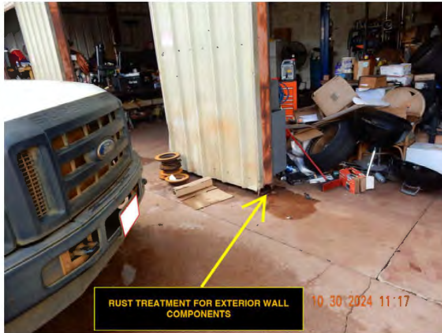
Figure 68. Rusting exterior wall steel components (DSCN3760).
