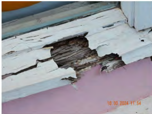
Figure 42. Termite damage to window seal, typical (DSCN3971).
