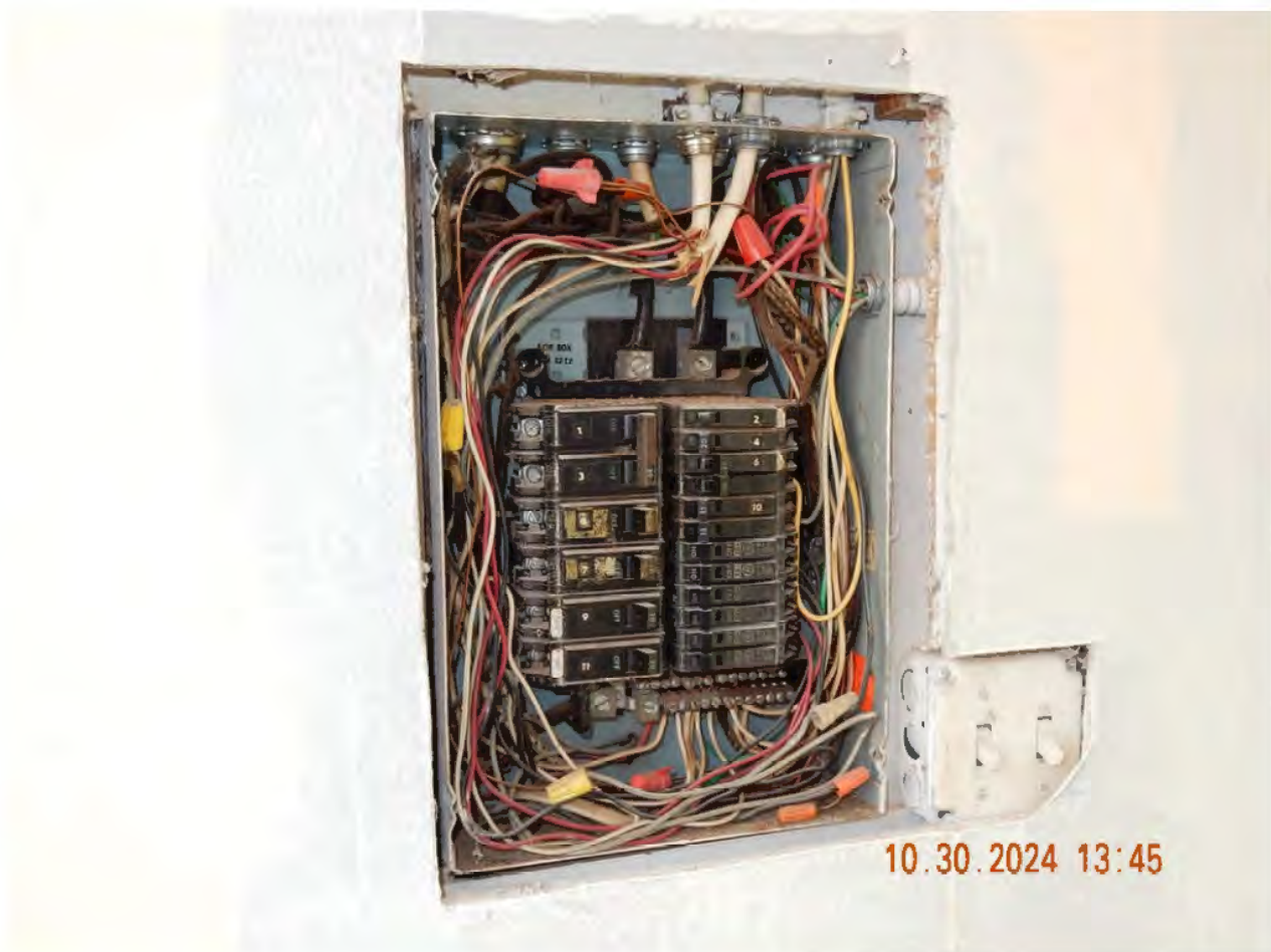
Figure 52. Electrical panel in Building #1, south wall (DSCN4079).
