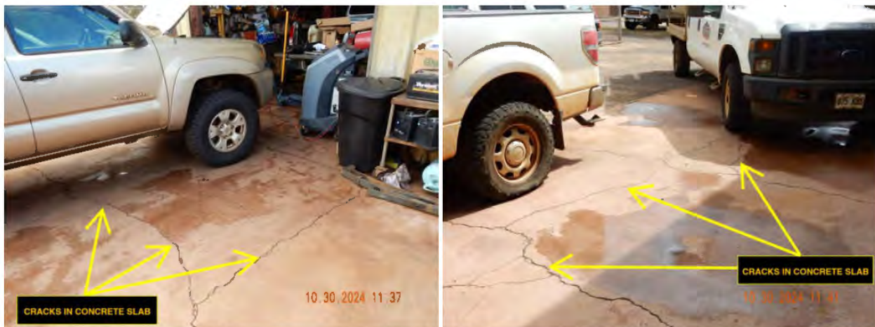
Figure 69 & 70. Cracks in concrete slab (DSCN3856 & DSCN3871).
