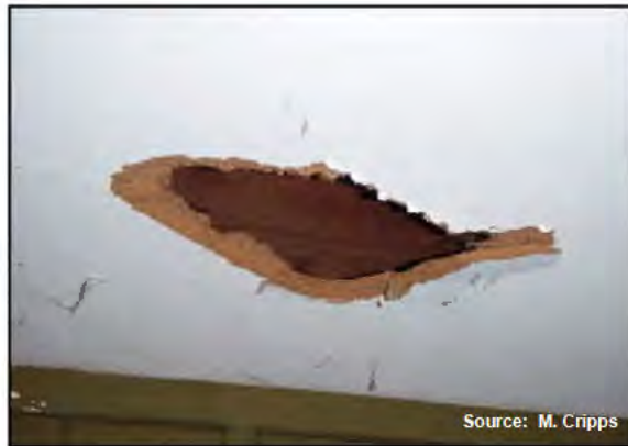
A canec panel that is broken. Note the characteristic fibrous texture and brownish color.
