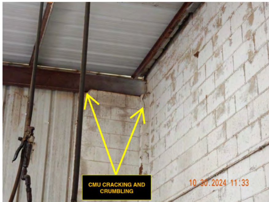
Figure 72. CMU cracking and crumbling at a structural point (DSCN3828).
