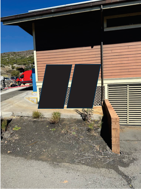
Fig. 3, Closer rendering of installed solar collectors. New exterior piping (not depicted) would consist of a single, insulated copper pipe connecting the collectors to system in Mechanical Room.
