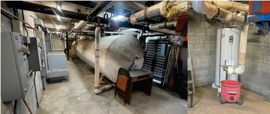
Fig. 4, (Left) 1900 Hot water insulated holding tank and (right) electric water heater.
