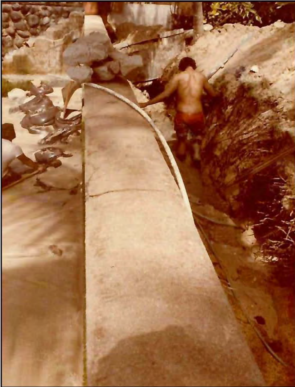
Note: In-line photo of original seawall with trenching for new revetment to be built mauka of the seawall.
