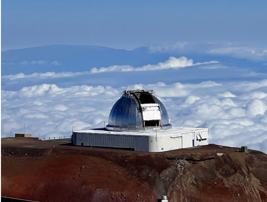
Figure 1: View of IRTF and eastern face of Pu'u'hau'oki. Evidence of erosion shown in precipitation run-off marks. Existing retaining wall appears as a slightly curved black line near the top of the pu'u.
