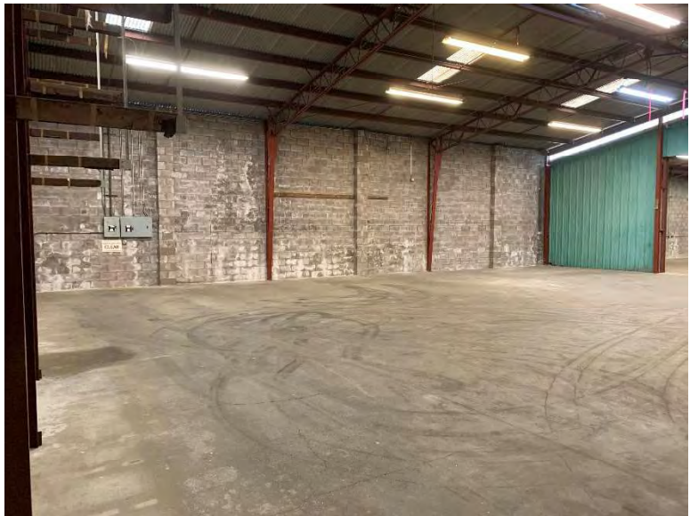
LEFT SIDE BAYS 3 & 4 WITH ELECTRICAL PANEL FOR BAY 5
