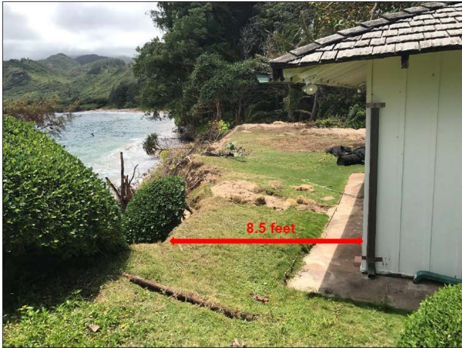
Figure 13 Greig single-family home 8.5 feet from the erosion scarp, TMK (1) 5-5-002:088
