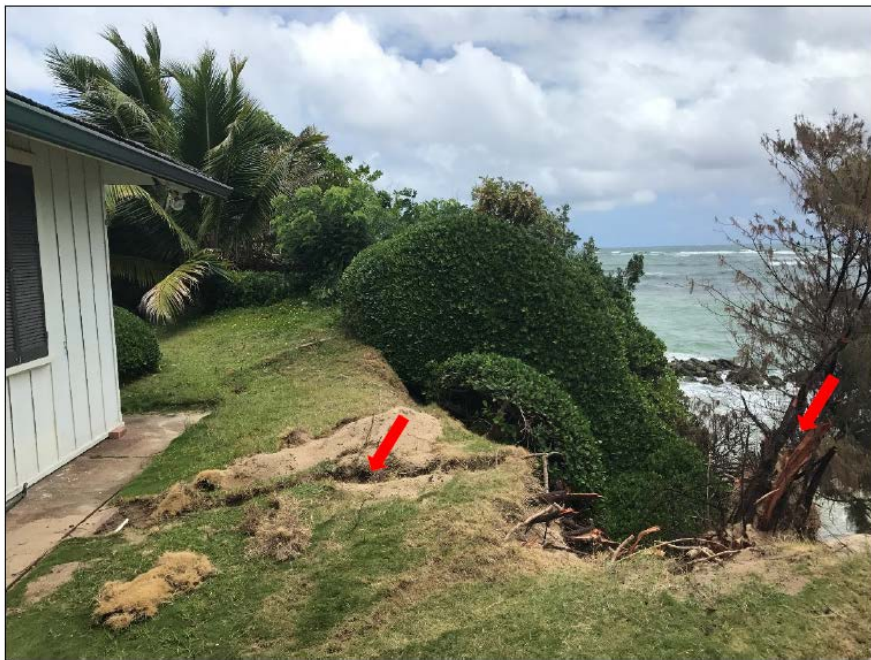
Figure 14 Collapsed trees and damaged water infrastructure, TMK (1) 5-5-002:019
