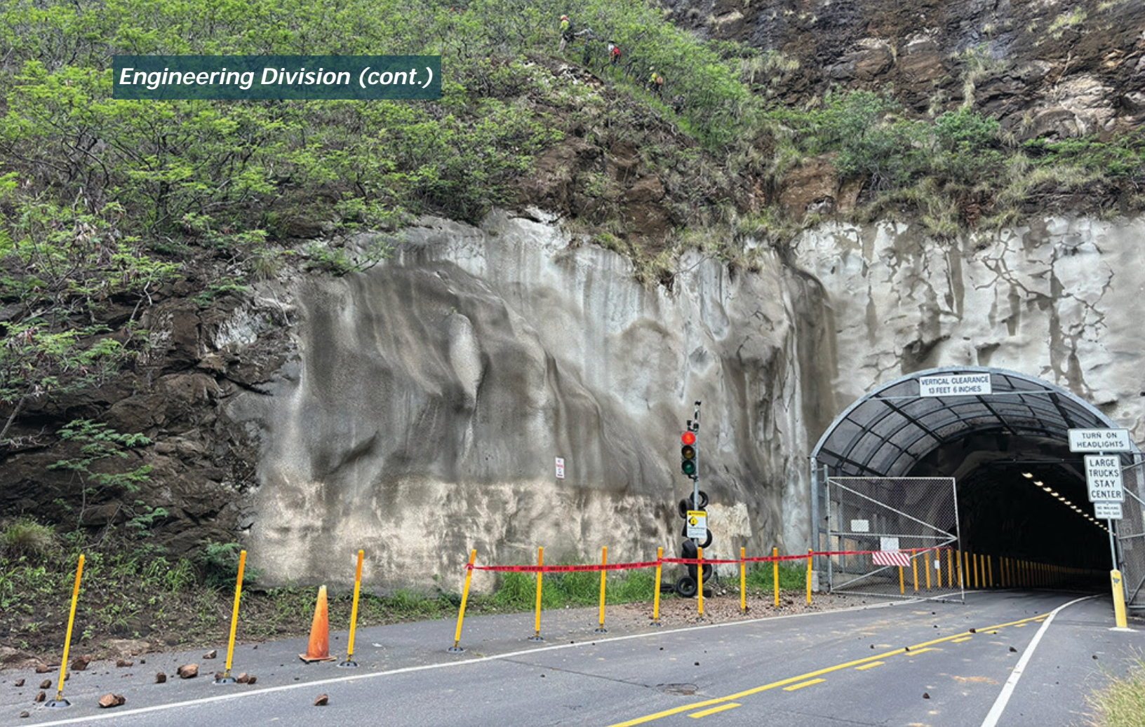
Entry to Diamond Head State Monument before construction, showing large rockfall cliffs, rock debris on the ground, and rusted metal cage needing replacement.
