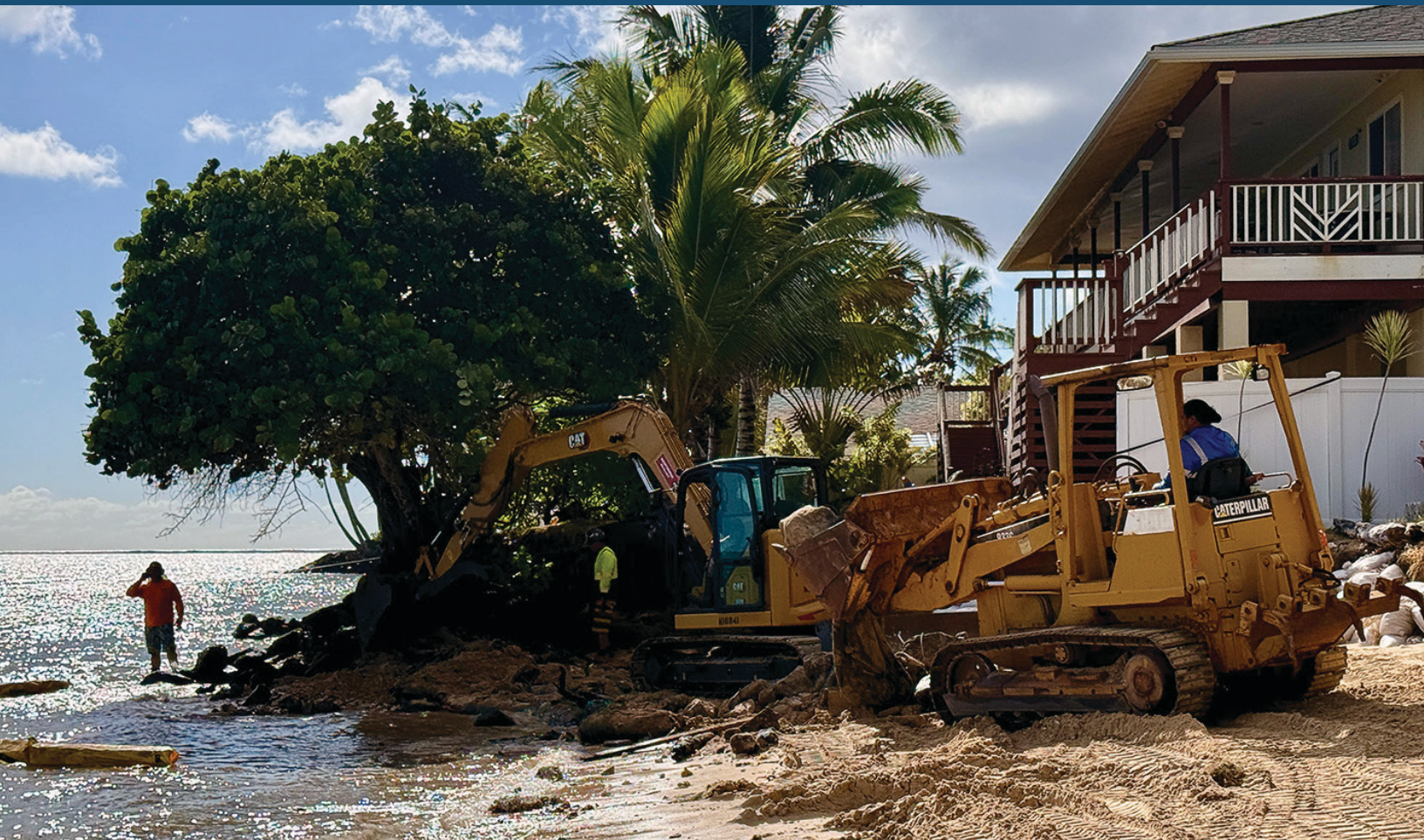
A contractor with the Office of Conservation and Coastal Lands prepares to remove an unauthorized seawall from state land at Punalu'u, O'ahu, September 8, 2025.
