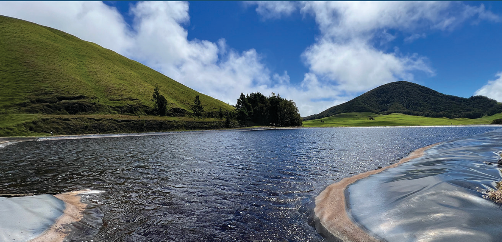
Photo from a dam inspection conducted by Engineering Division staff at the Punawai Reservoir near Waimea town on Hawai'i Island.
