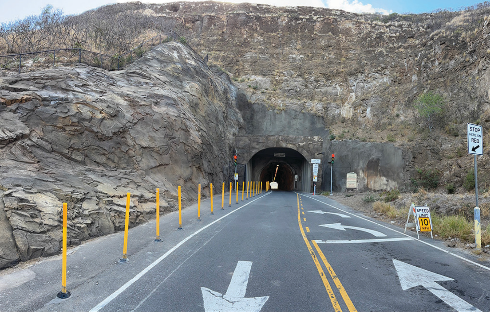
Entry to Diamond Head State Monument after construction, showing fresh shotcrete work, new concrete tunnel structure and no rockfall debris.
