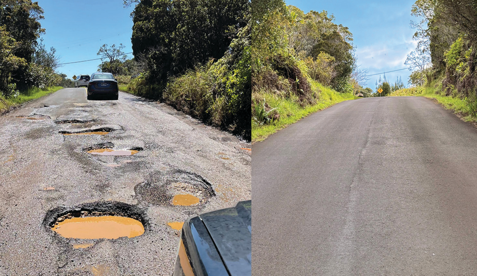
Before and after photos of the Kōkeʻe State Park access road repairs between the Kalalau Lookout and Puʻu o Kila Lookout, Kauaʻi, Hawaiʻi, completed in December 2025.
