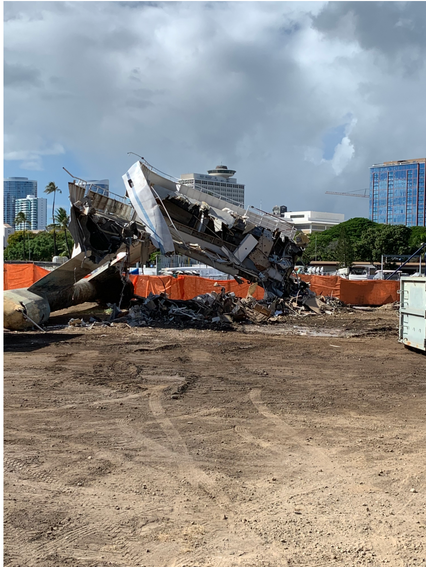
Exhibit T-3: Vessel destruction underway at RP 157 (Parcel B), Ala Wai Small Boat Harbor, with Waikīki skyline and harbor visible in the background. Orange safety fencing surrounds the debris. Multiple vessels have been safely destroyed on this site. Question: is this an essential harbor management function?
