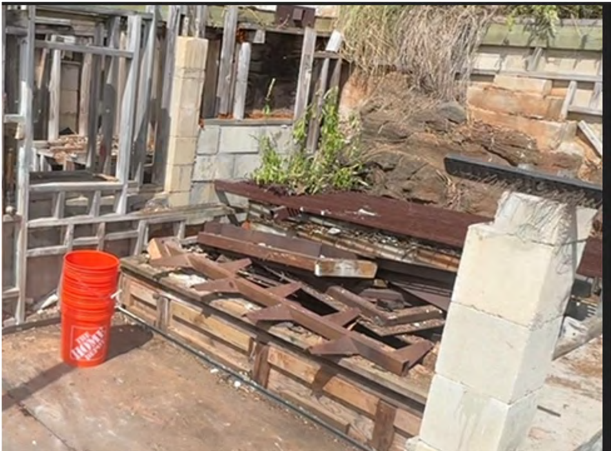
Shed Before (Top Photo) and After (Bottom Photo) Additional Removal and Cleanup
