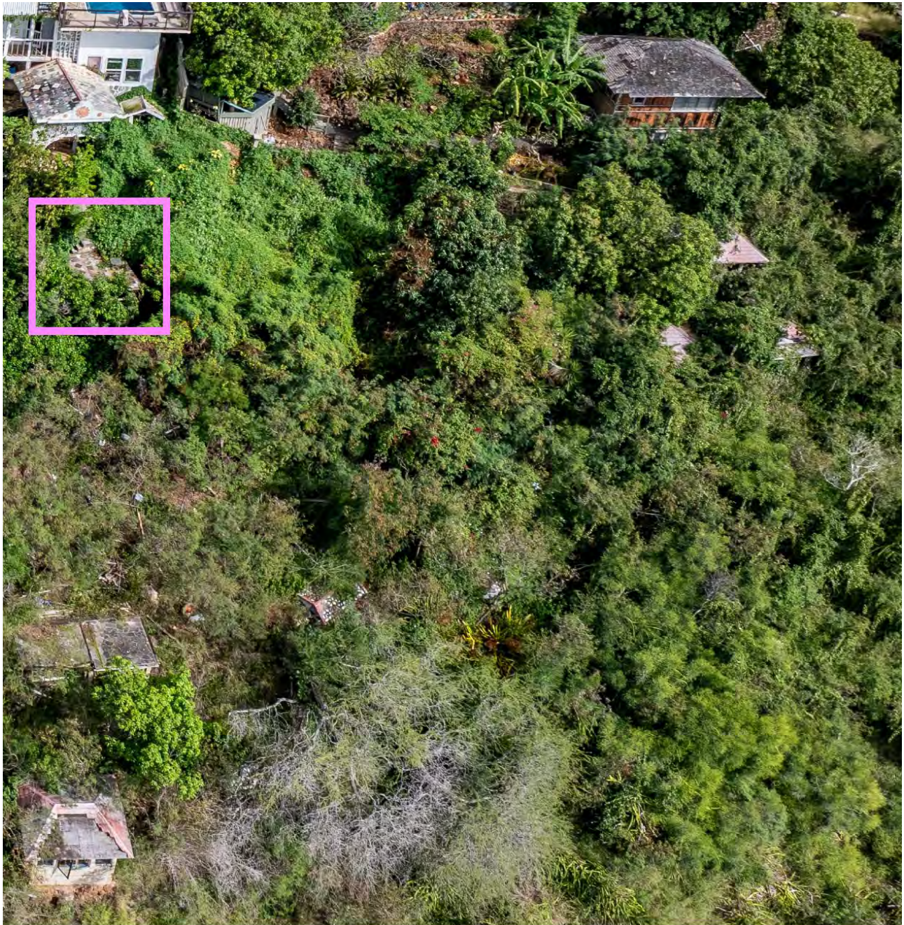
From Exhibit 3 Portion of Photo noted as Appendix 1, Page 7. Purple square is of a deck that was removed. This photo is from 2025 and illustrates what is believed to be remnants of authorized picnic shelters, lots of vegetation, and debris on the property.
