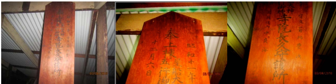
Photos taken by Jake Bierman, April 3, 2018, during inspection of Hakalau Jodo Mission buildings
