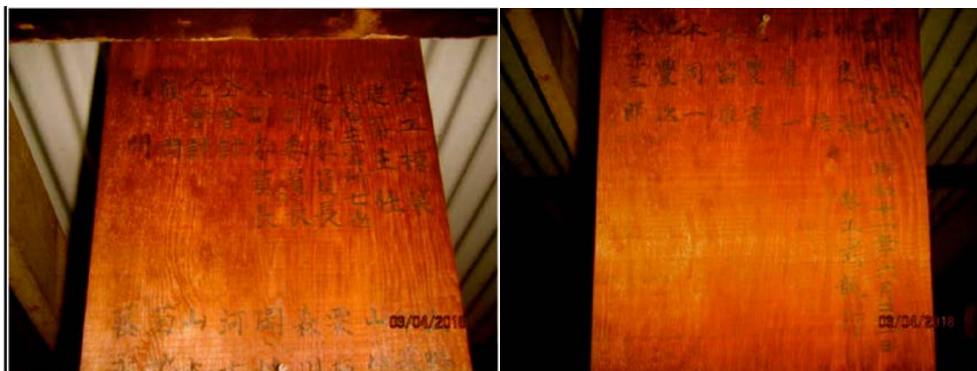
Photos taken by Jake Bierman, April 3, 2018, during inspection of Hakalau Jodo Mission buildings
