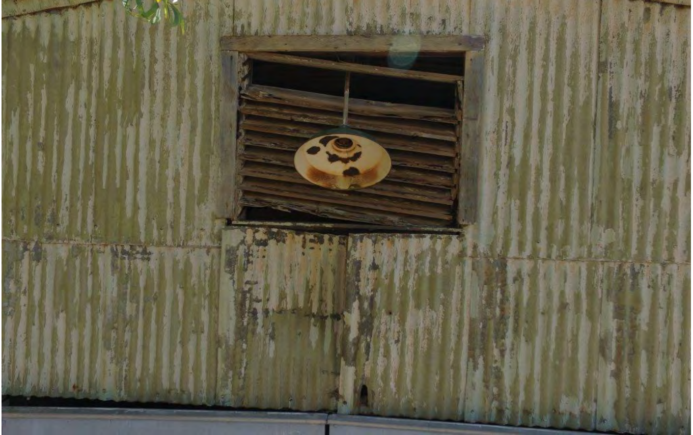
Photo 6. View of louvered window vent above doorway in north bulkhead wall, Quonset Hut 33, O’ahu Urban Garden Center, camera facing southwest. Photo by Carroll Cox. 2015.
