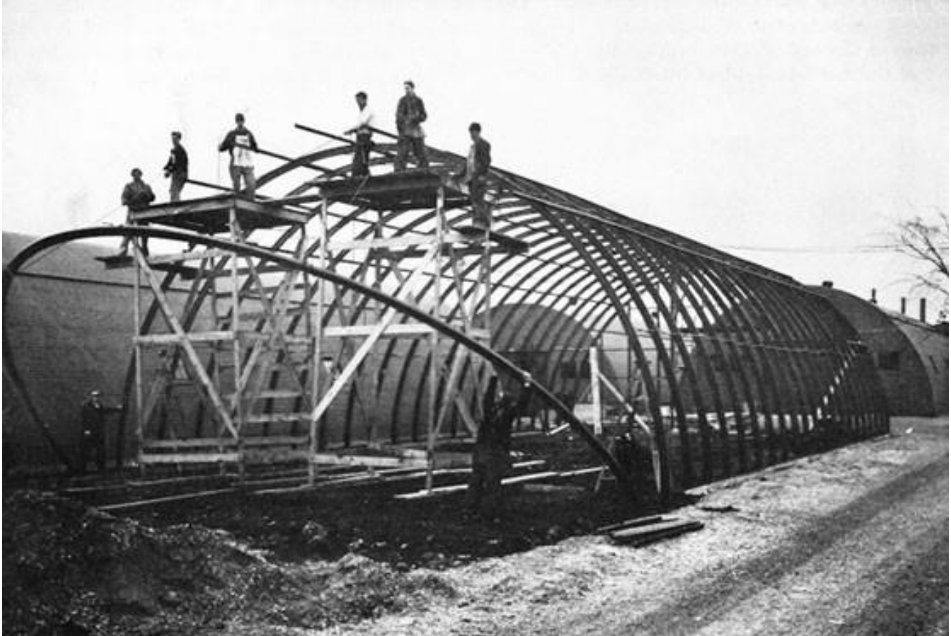
Figure 29. An SSAR 40 Quonset hut under construction for use as a school at the Central Spare Parts Warehouse in Joliet, Illinois. Note the frame of I-shaped ribs with additional support provided by ties bars and longitudinal ribs at the roof.
