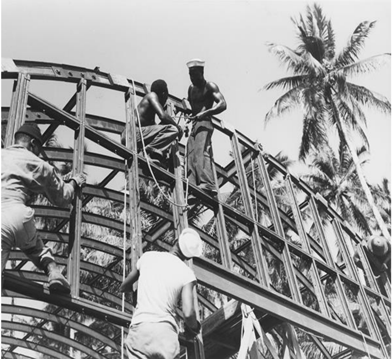
Figure 9. "Members of the 34th NCB erecting a 40 x 100 foot Quonset hut warehouse at Halavo Seaplane Base, Florida Island, Solomon Islands, Sept. 19, 1943." Source: Frank A. Blazich, Jr., "Building for a Nation and Equality: African American Seabees in World War II," http://seabeesmagazine.navylive.dodlive.mil/2014/03/06/building-for-a-nation-and-equality-african-american-seabees-in-world-war-ii/ , crediting US Navy Seabee Museum.
