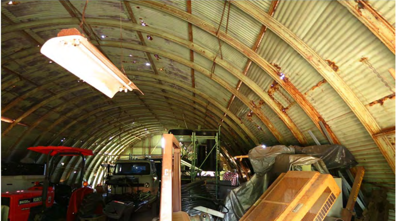
Photo 7. Interior view of Quonset Hut 33 in the Urban Garden, University of Hawai'i at Mānoa College of Tropical Agriculture and Human Resources, camera facing southwest. From NAVFAC-HI. 2014.
